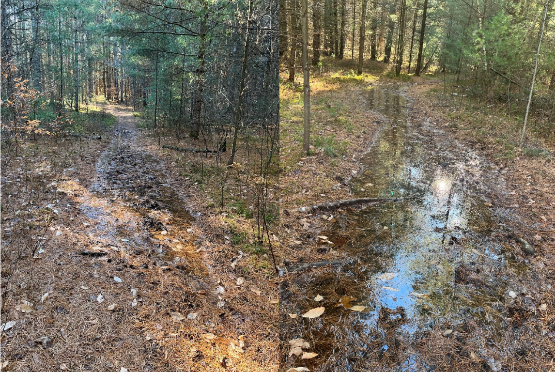
Images: Examples of locations along Frost Pocket Trail where turnpike will be installed.
