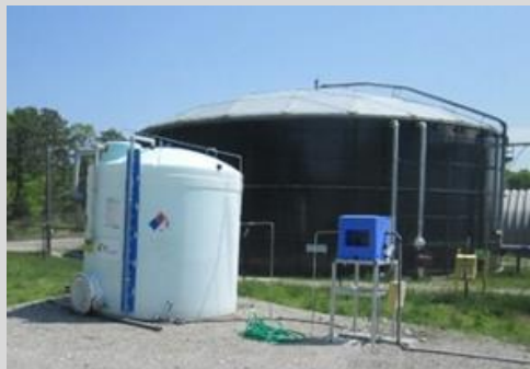
Hydrogen Peroxide (H 2 O 2 ) dosing system
