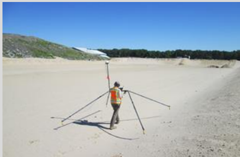
Electrical check for leaks in newly installed landfill liner in Cell 6 Phase XI prior to obtaining certification for construction, and commencing landfilling activities
