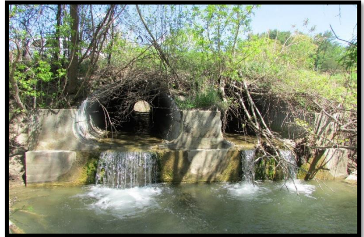
Culverts such as this these can constrict the natural flow of the stream, have a perched outlet that only strong swimmers can jump and contain no natural streambed. Many culverts and dams fragment
