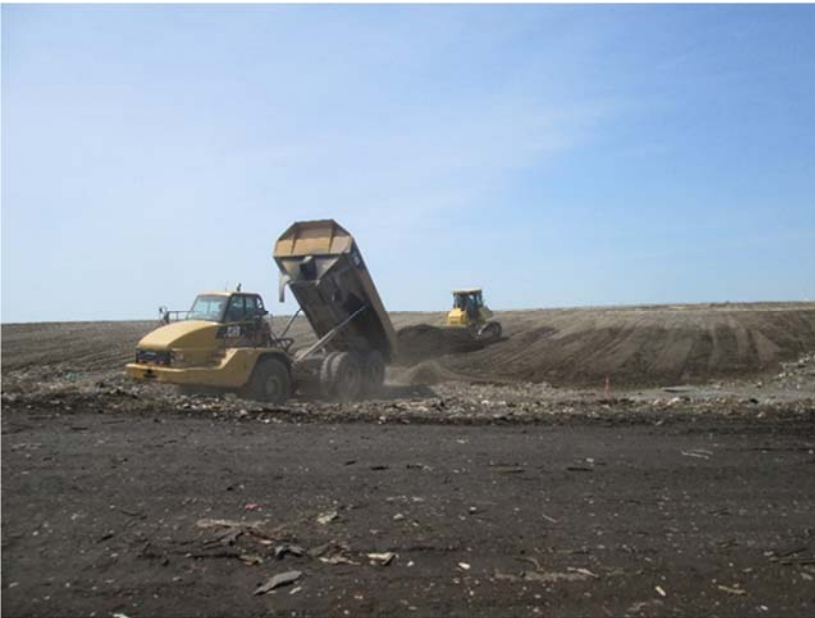
Smooth grading at the topside of the landfill with layer of additional soil
