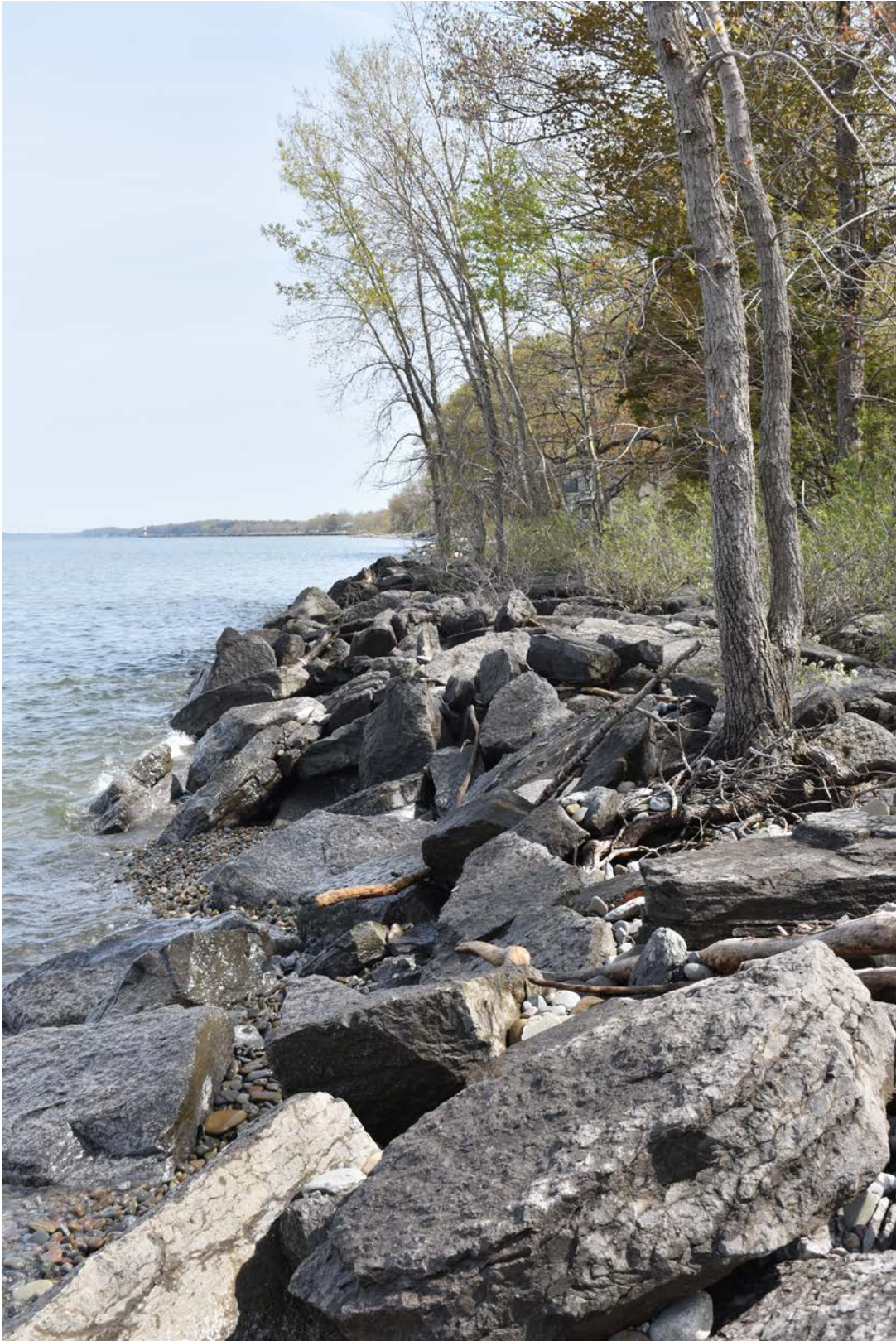
Photo 2. Shoreline protection along the banks of Selkirk Shores State Park in the 1960's and 1970's
