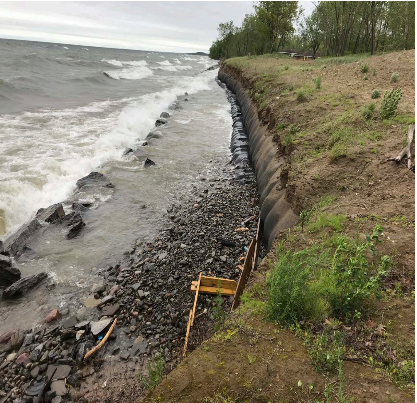
Photo 1. Existing Conditions: Sand placed during the 2017 construction to protect this natural dune structure has been affected by more recent high water levels, and has exposed trap bags. If these trap bags fail, the entire dune will be in jeopardy.
