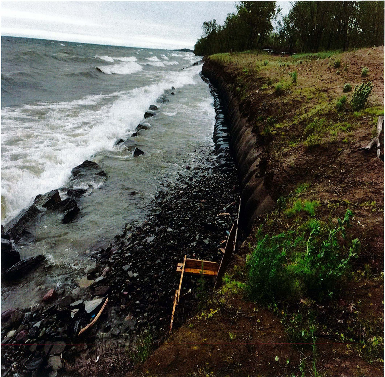
Photo 1. Existing Conditions: Sand placed during the 2017 construction to protect this natural dune structure has been affected by more recent high water levels, and has exposed trap bags. If these trap bags fail, the entire dune will be in jeopardy.
