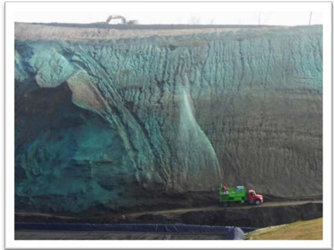
DEC requires hydroseeding at the Dunn facility to stabilize the sand, reducing offsite dust issues.
