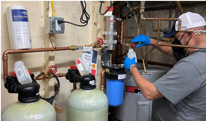
Point of Entry Treatment System and Maintenance Sampling
