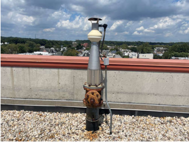
Photo 1: View of typical operational SSDS fan unit on the roof.
