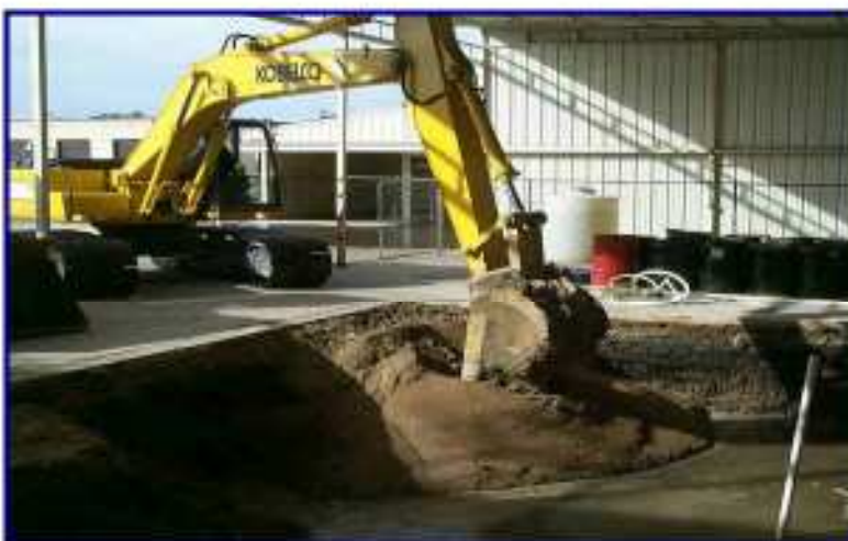
Photo 2. Picture of excavator leveling EHC and sand that were mixed together prior to placement into the excavated area
