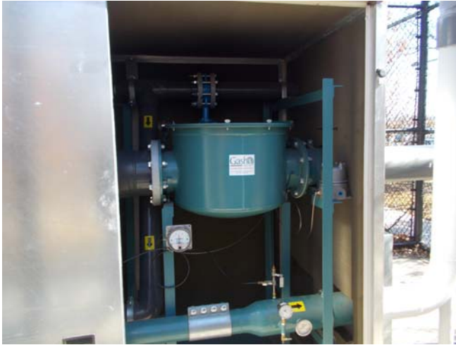
Photo 1: View of the SSDS fan unit.
