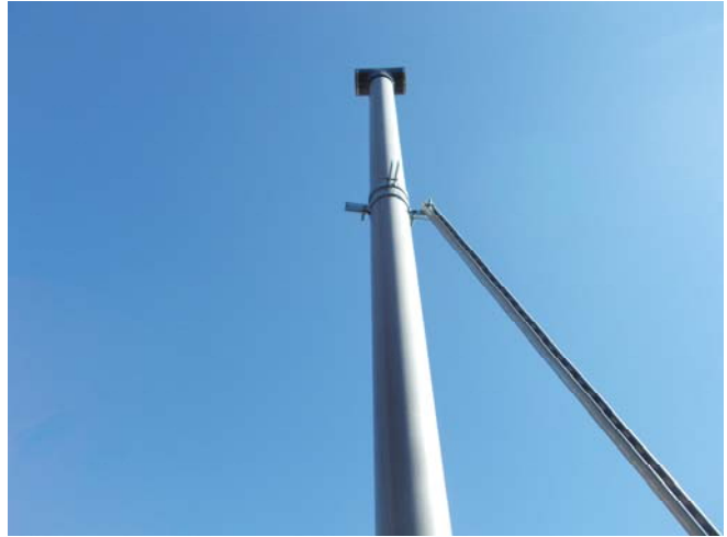
Photo 2: View of SSDS vent stack.
