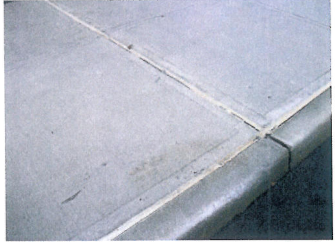
Photo 14: View of noticeable separation between side walk and its edge by the artificial turf on North side.
