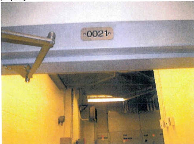
Photo 5: View of entrance to Room # 0021 which has floor cracks.
