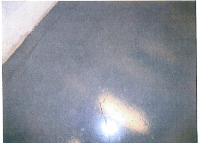
Photo 6: View of hairline cracks in Room # 0021 floor hair.
