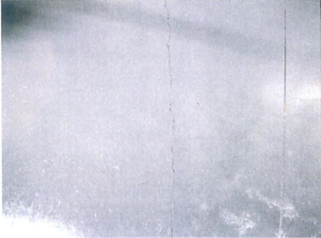
Photo 7: View of hairline cracks in room # 0021 floor.
