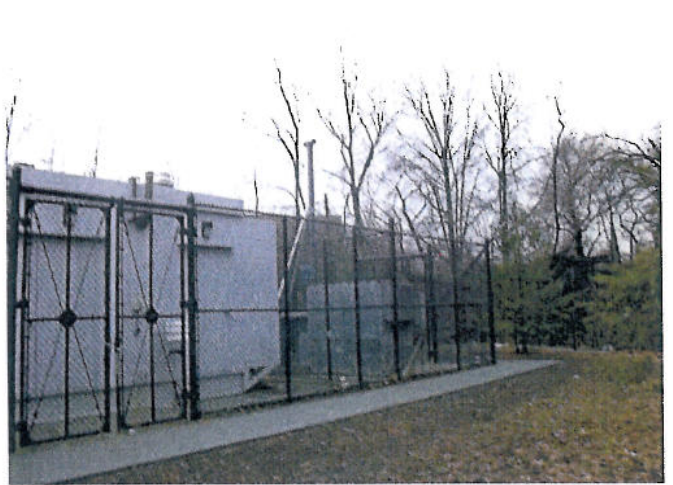
Photo 4: View of blower unit in the southern portion of the property.
