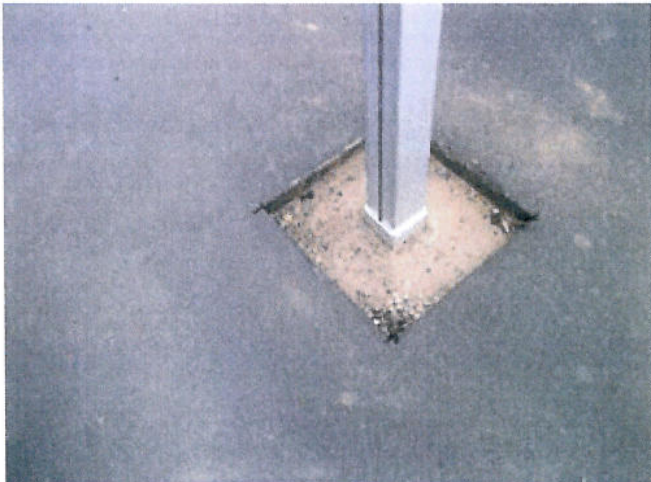
Photo 11: View of volleyball court (spot cutting of the paved area to erect the net pole).
