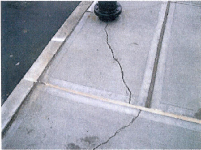
Photo 9: View of sidewalk cracks by district 75/Q233 exit.
