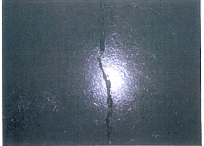
Photo 8: View of a minimum of 1/4" crack in Room 0021.
