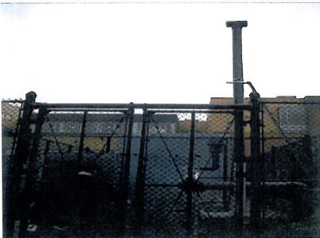
Photo 3: View of blower unit in the southern portion of the property.
