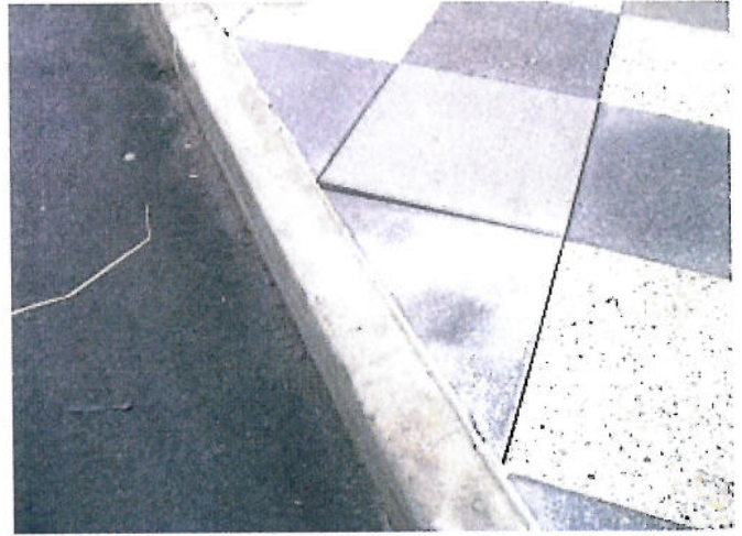
Photo 16: View of uneven side walk floor tiles by Queens Metropolitan HS entrance.
