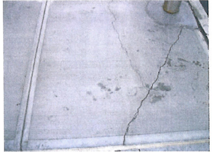
Photo 10: View of sidewalk cracks by district 75/Q233.
