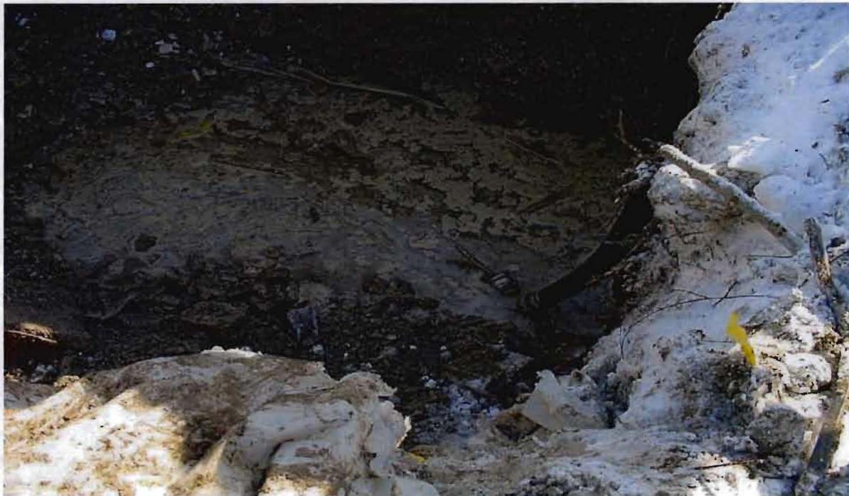
Stormwater pumped out of excavation at the beginning of the 3 January 2001 remedial activities.
