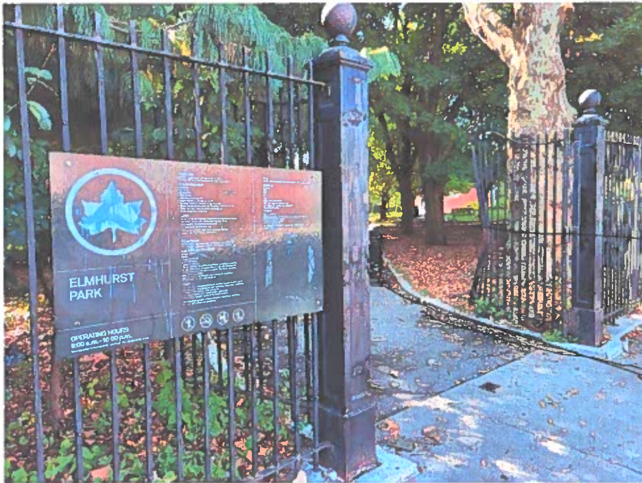
#1, NE entrance fence rusted; park signage defaced, gate damaged
