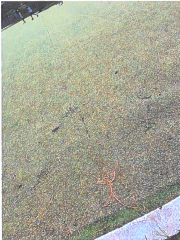
#8, Synthetic Turf, gaps in surface appearing
