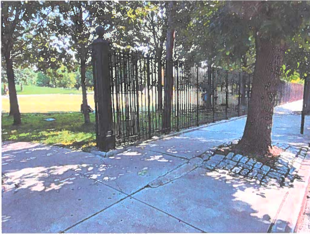
#8, Root damage to sidewalk and entrance gate column (leaning)
