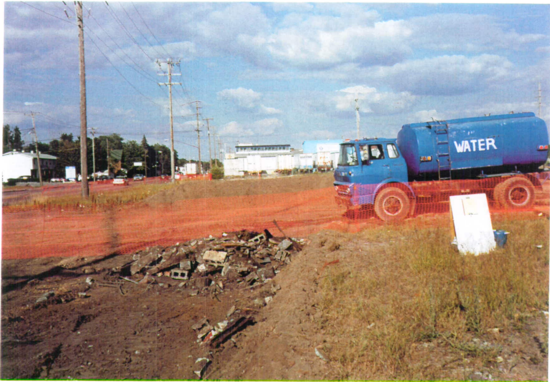
Debris deposit in the entrance excavation, July 13, 1999
