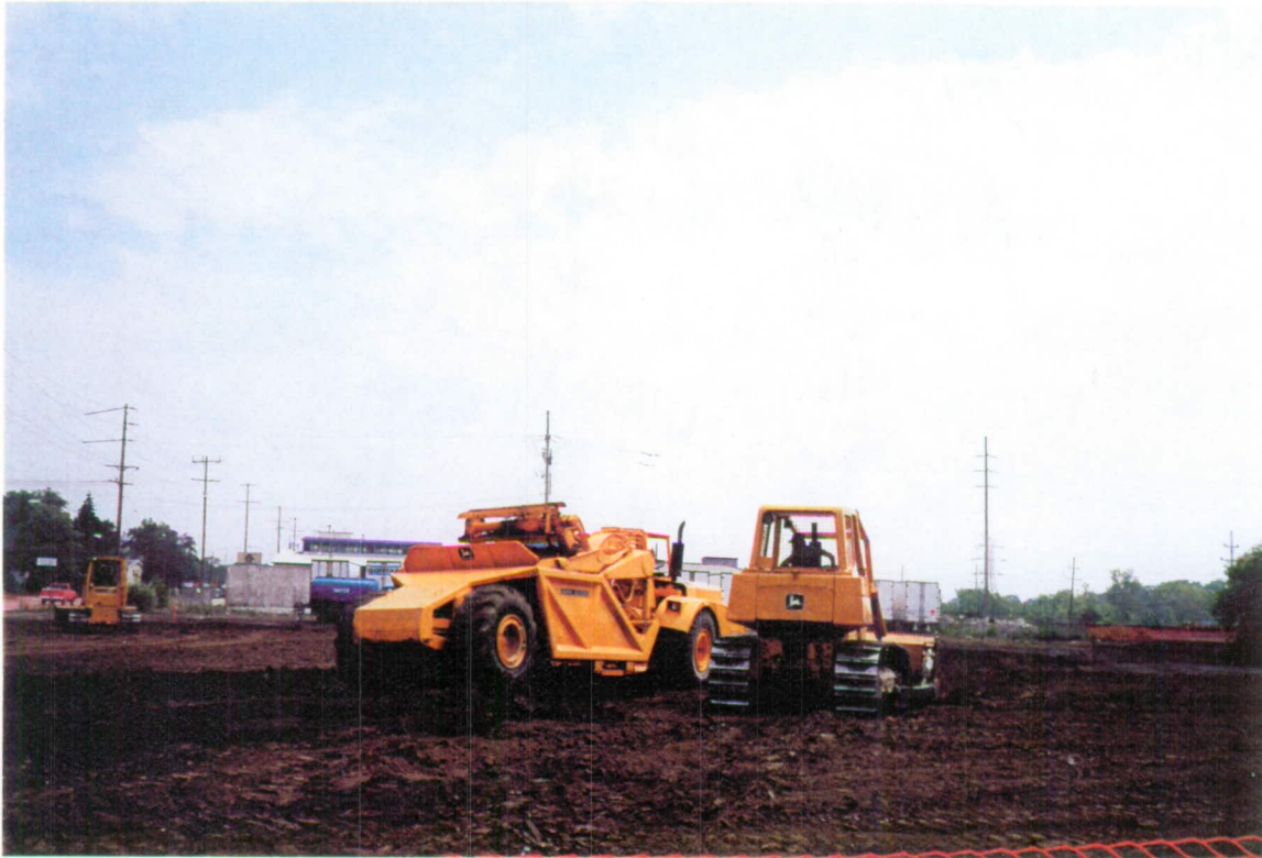
Two bulldozers and a Pan moving the topsoil from the new entrance at north west going toward the south-east corner, July 15, 1999
