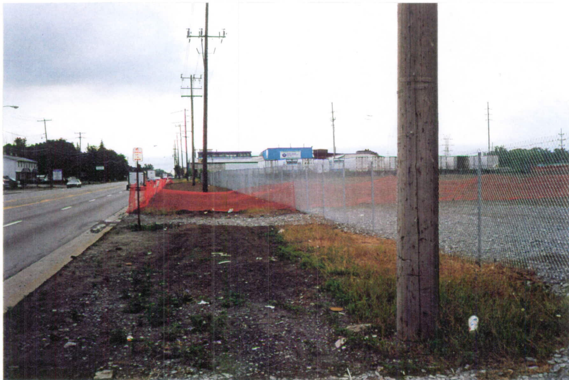
After rake out of new topsoil Safety fence reinstalled because new fence is not complete, July 16, 1999
