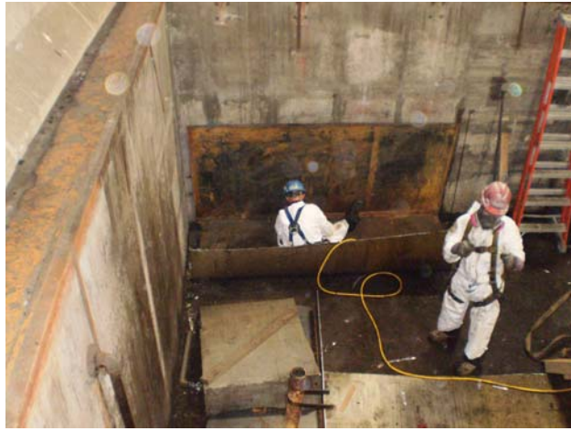
082009-01 Emergency Dump Tank.JPG
