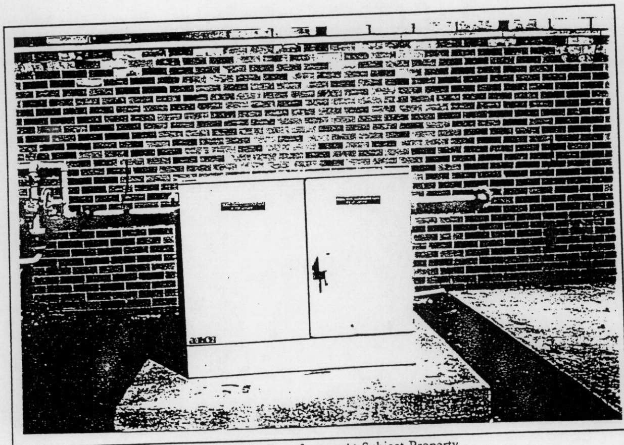
Photograph 8: Transformer At Subject Property
