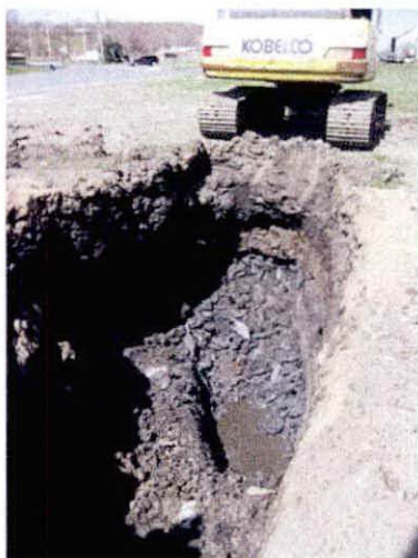
Groundwater collected in excavation
