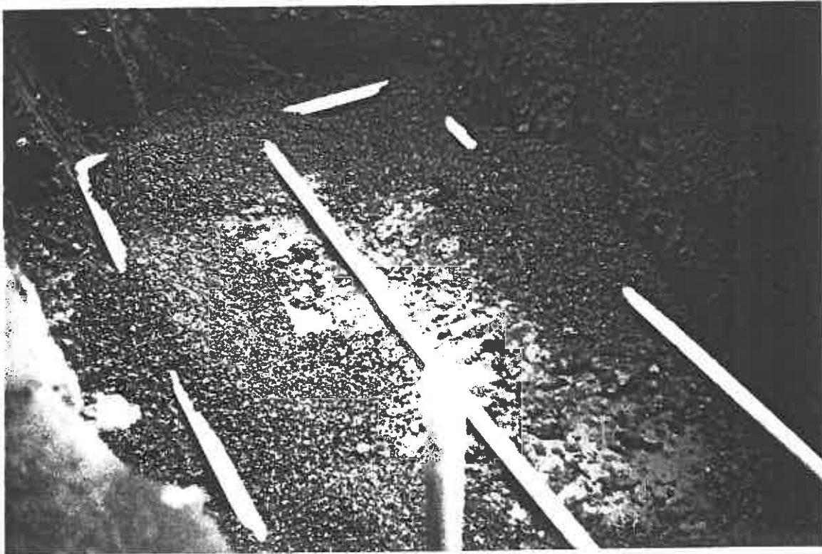
Groundwater Collection Pipes in Pit
