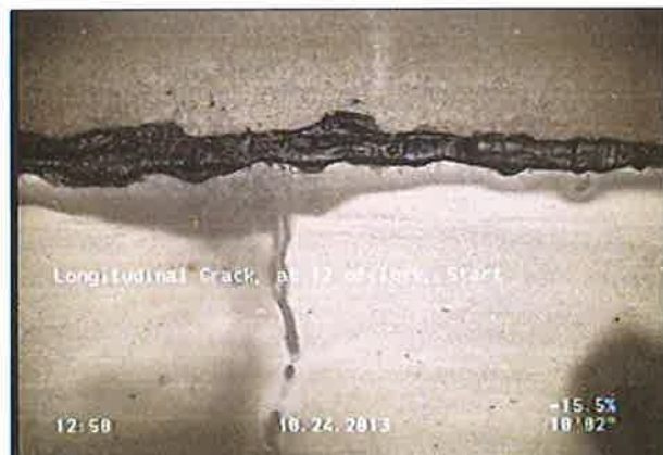
Photo: 10-11-18_10-10-6_2_24102013_125509_A.JPG Longitudinal Crack, at 12 o'clock, Start
