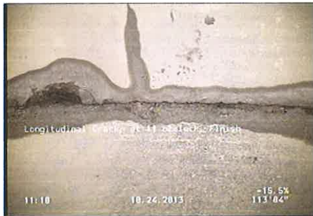
Photo: 10-9_10-10-6_14_24102013_111553_A.JPG Longitudinal Crack, at 11 o'clock, Finish
