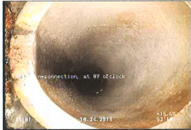
Photo: 10-9_10-10-6_6_24102013_110627_A.JPG break-in-connection, at 09 o'clock
