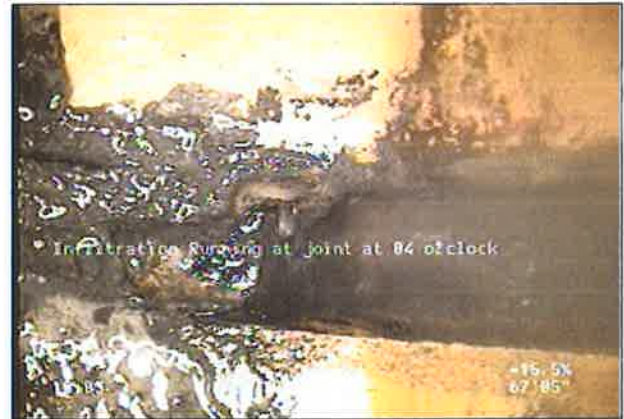
Photo: 10-1_10-2-16_8_23102013_100842_A.JPG Infiltration Running at joint at 04 o'clock
