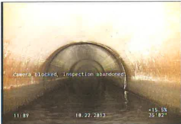
Photo: MH-1_2-16_5_22102013_111421_A.JPG camera blocked, inspection abandoned
