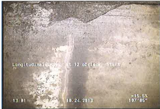
Photo: 10-11-18_10-10-6_9_24102013_130651_A.JPG Longitudinal Crack, at 12 o'clock, Start
