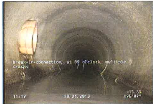
Photo: 10-9_10-10-6_18_24102013_112450_B.JPG break-in-connection, at 09 o'clock / multiple cracks
