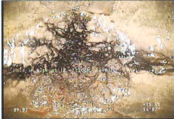
Photo: 10-3_10-4_4_23102013_090806_A.JPG Hole in pipe at 12 o'clock / seeping
