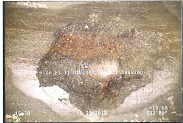
Photo: 2-16_MH-3_36_22102013_153553_A.JPG Hole in pipe at 11 o'clock / repair leaking
