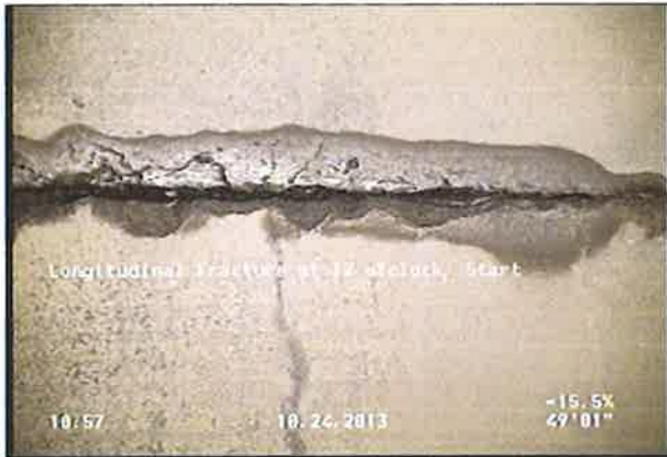
Photo: 10-9_10-10-6_5_24102013_110253_A.JPG Longitudinal Fracture at 12 o'clock, Start
