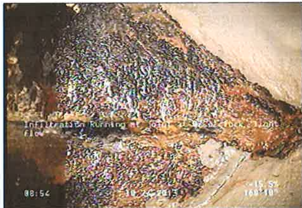
Photo: 10-8-21_10-9_8_24102013_085931_A.JPG Infiltration Running at joint at 07 o'clock / light flow
