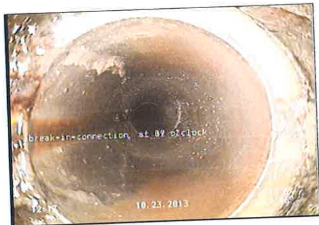
Photo: 10-5-7_10-7-21_6_23102013_122208_A.JPG break-in-connection, at 09 o'clock
