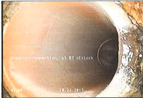
Photo: 10-9_10-10-6_12_24102013_111412_A.JPG break-in-connection, at 03 o'clock
