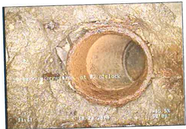
Photo: 10-6_10-5-7_6_23102013_114705_A.JPG break-in-connection, at 02 o'clock
