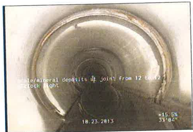
Photo: 10-5-7_10-7-21_5_23102013_122130_A.JPG scale/mineral deposits at joint from 12 to 12 o'clock light
