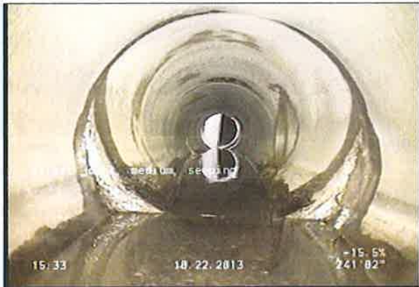
Photo: 2-16_MH-3_39_22102013_153859_B.JPG offset joint, medium / seeping
