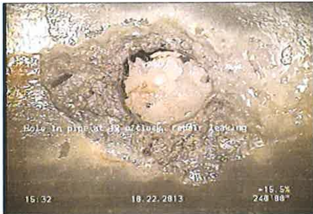
Photo: 2-16_MH-3_38_22102013_153733_A.JPG Hole in pipe at 12 o'clock / repair leaking
