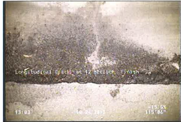
Photo: 10-11-18_10-10-6_10_24102013_130825_A.JPG Longitudinal Crack, at 12 o'clock, Finish
