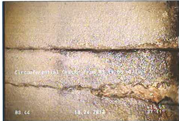
Photo: 10-8-21_10-9_3_24102013_084918_A.JPG Circumferential Crack, from 03 to 05 o'clock
