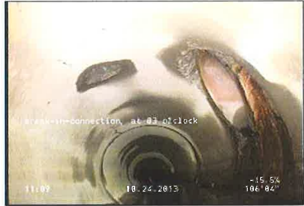
Photo: 10-9_10-10-6_12_24102013_111433_B.JPG break-in-connection, at 03 o'clock
