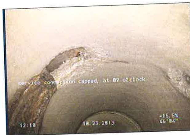
Photo: 10-5-7_10-7-21_7_23102013_122407_B.JPG service connection capped, at 09 o'clock
