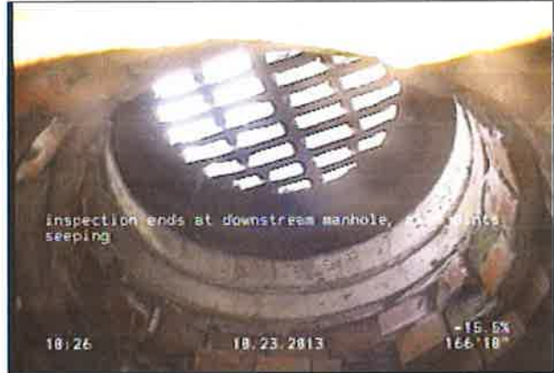
Photo: 10-1_10-2-16_25_23102013_103125_A.JPG inspection ends at downstream manhole / all joints seeping
