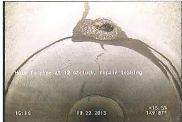
Photo: 2-16_MH-3_22_22102013_151913_B.JPG Hole in pipe at 12 o'clock / repair leaking
