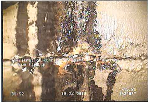
Photo: 10-8-21_10-9_7_24102013_085718_A.JPG Infiltration Running at joint at 07 o'clock / medium flow
