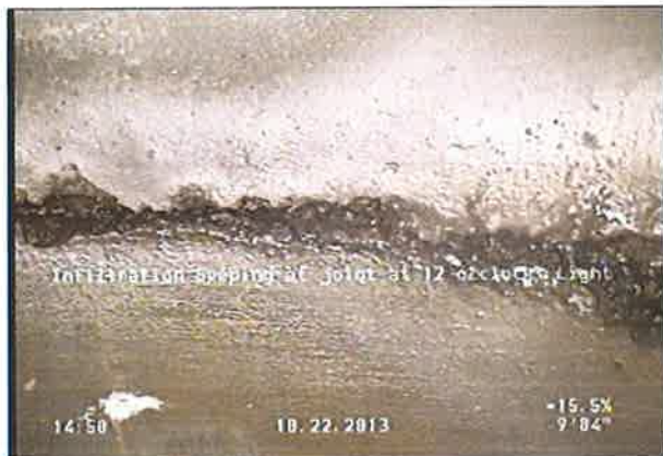
Photo: 2-16_MH-3_2_22102013_145515_A.JPG Infiltration Seeping at joint at 12 o'clock / Light
