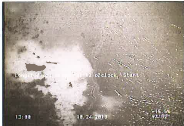
Photo: 10-11-18_10-10-6_7_24102013_130510_A.JPG Longitudinal Crack, at 12 o'clock, Start
