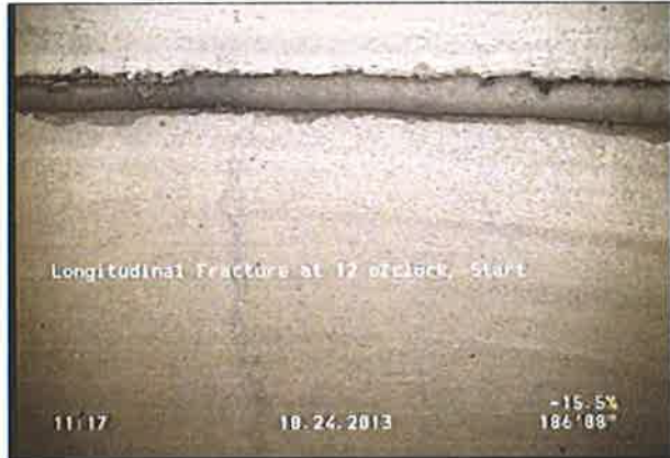
Photo: 10-9_10-10-6_16_24102013_112259_A.JPG Longitudinal Fracture at 12 o'clock, Start
