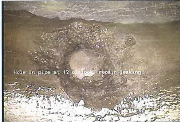
Photo: 2-16_MH-3_43_22102013_154253_A.JPG Hole in pipe at 12 o'clock / repair leaking
