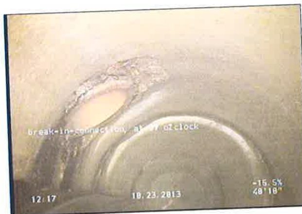
Photo: 10-5-7_10-7-21_6_23102013_122225_B.JPG break-in-connection, at 09 o'clock
