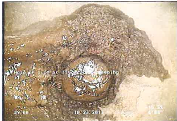
Photo: 10-3_10-4_2_23102013_090558_A.JPG Hole in pipe at 11 o'clock / seeping
