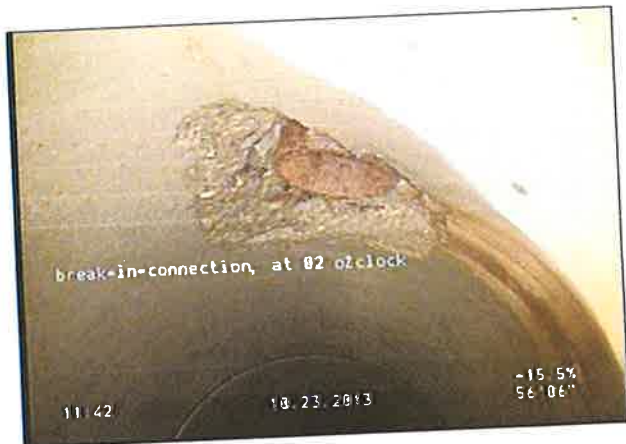
Photo: 10-6_10-5-7_6_23102013_114717_B.JPG break-in-connection, at 02 o'clock
