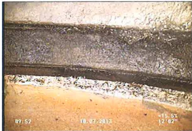
Photo: 10-1_10-2-16_2_23102013_095756_A.JPG separated joint slight
