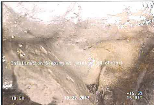
Photo: MH-1_2-16_2_22102013_110401_A.JPG Infiltration Seeping at joint at 08 o'clock
