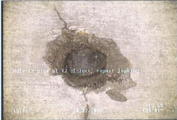
Photo: 2-16_MH-3_24_22102013_152118_A.JPG Hole in pipe at 12 o'clock / repair leaking
