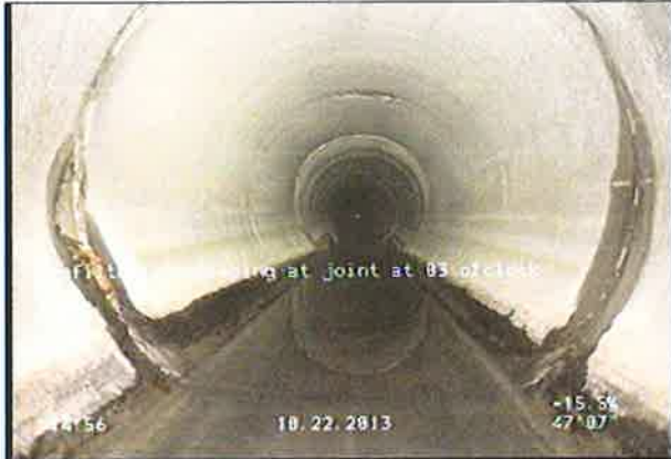
Photo: 2-16_MH-3_6_22102013_150116_A.JPG Infiltration Seeping at joint at 03 o'clock
