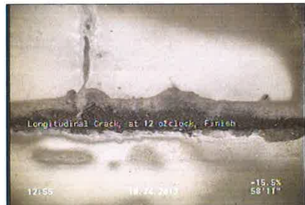
Photo: 10-11-18_10-10-6_3_24102013_130013_A.JPG Longitudinal Crack, at 12 o'clock, Finish
