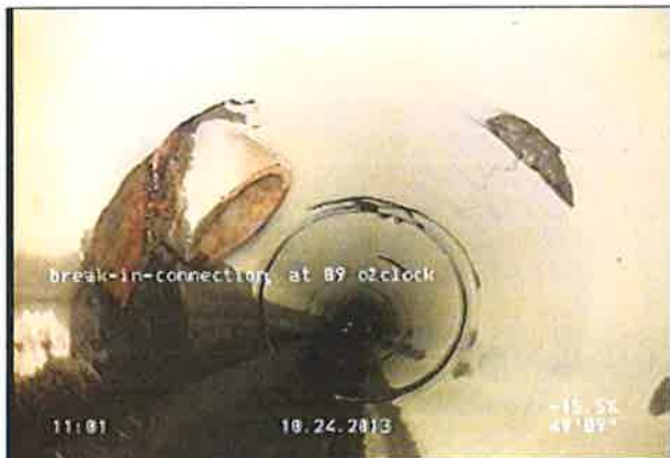
Photo: 10-9_10-10-6_6_24102013_110648_B.JPG break-in-connection, at 09 o'clock
