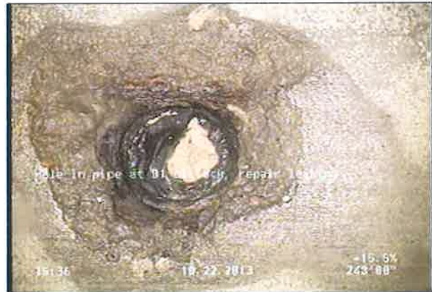
Photo: 2-16_MH-3_41_22102013_154128_A.JPG Hole in pipe at 01 o'clock / repair leaking
