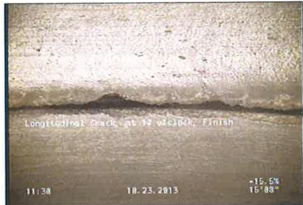
Photo: 10-6_10-5-7_3_23102013_113546_A.JPG Longitudinal Crack, at 12 o'clock, Finish
