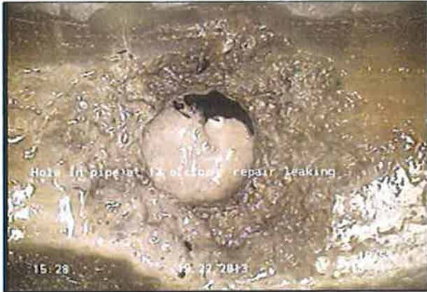
Photo: 2-16_MH-3_34_22102013_153325_A.JPG Hole in pipe at 12 o'clock / repair leaking
