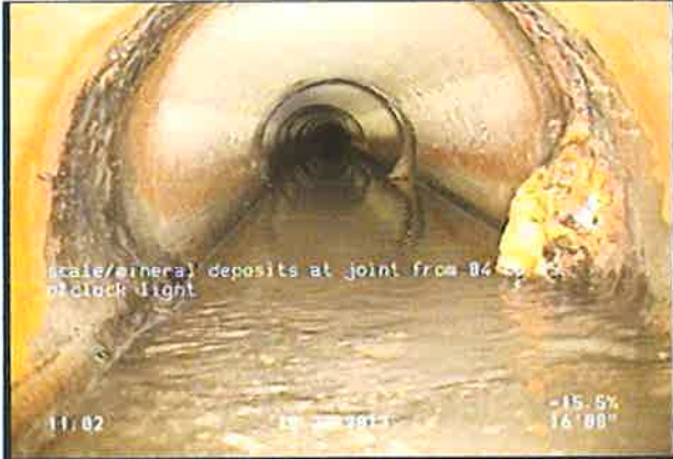
Photo: MH-1_2-16_3_22102013_110802_B.JPG scale/mineral deposits at joint from 04 to 05 o'clock light
