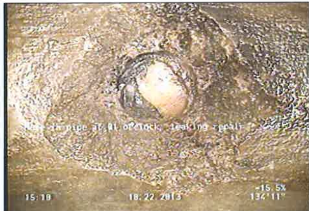
Photo: 2-16_MH-3_18_22102013_151516_A.JPG Hole in pipe at 01 o'clock / leaking repair
