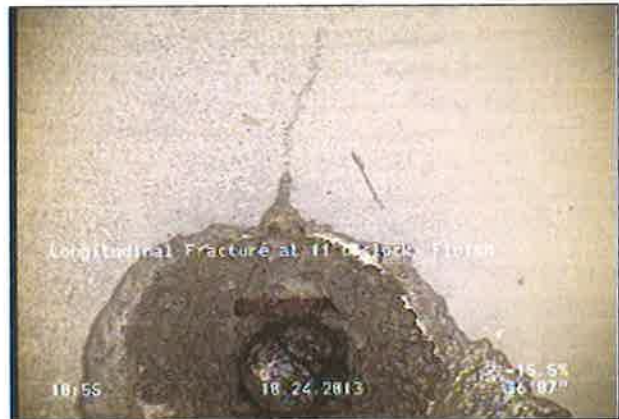
Photo: 10-9_10-10-6_3_24102013_110043_A.JPG Longitudinal Fracture at 11 o'clock, Finish
