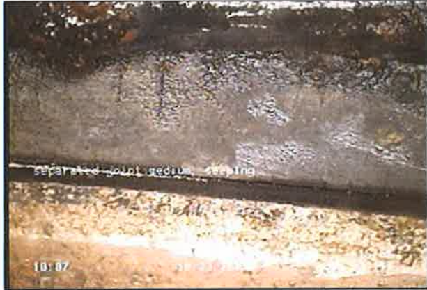
Photo: 10-1_10-2-16_11_23102013_101234_A.JPG separated joint medium / seeping
