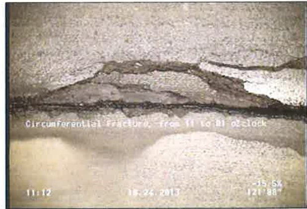
Photo: 10-9_10-10-6_15_24102013_111723_A.JPG Circumferential Fracture, from 11 to 01 o'clock
