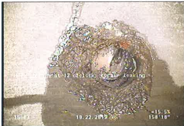
Photo: 2-16_MH-3_22_22102013_151902_A.JPG Hole in pipe at 12 o'clock / repair leaking
