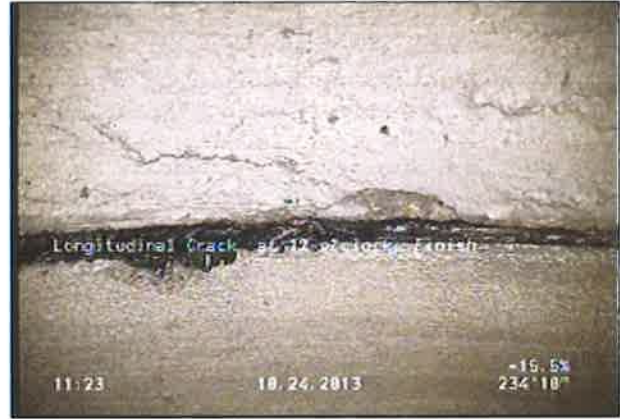
Photo: 10-9_10-10-6_20_24102013_112809_A.JPG Longitudinal Crack, at 12 o'clock, Finish
