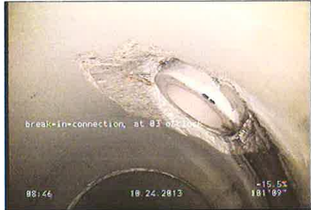
Photo: 10-8-21_10-9_4_24102013_085130_B.JPG break-in-connection, at 03 o'clock
