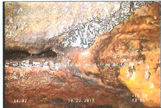
Photo: MH-1_2-16_3_22102013_110749_A.JPG scale/mineral deposits at joint from 04 to 05 o'clock light
