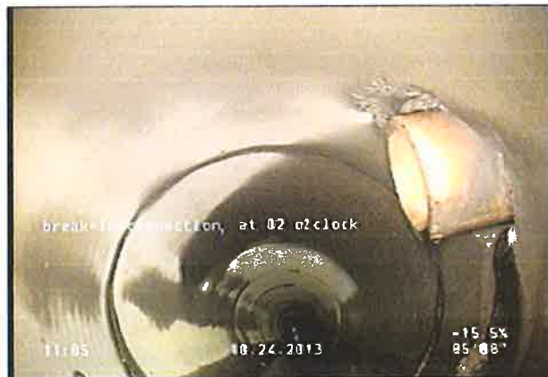
Photo: 10-9_10-10-6_11_24102013_111104_B.JPG break-in-connection, at 02 o'clock
