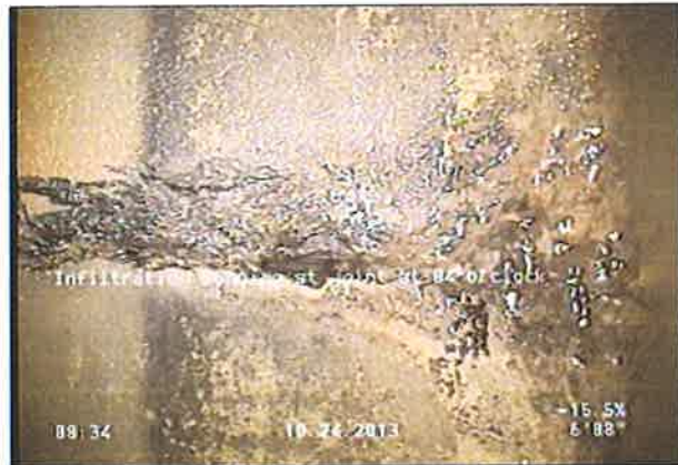
Photo: 10-8-21_10-9_2_24102013_083933_A.JPG Infiltration Running at joint at 04 o'clock
