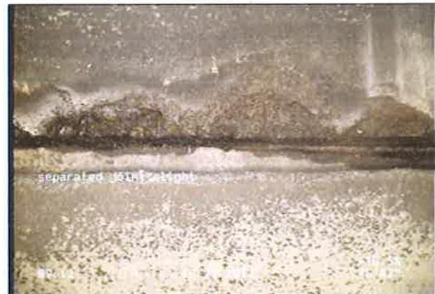
Photo: 10-3_10-4_11_23102013_091724_A.JPG separated joint slight
