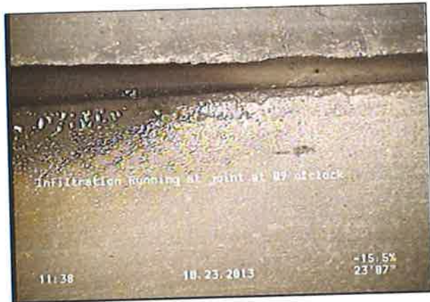
Photo: 10-6_10-5-7_4_23102013_114354_A.JPG Infiltration Running at joint at 09 o'clock
