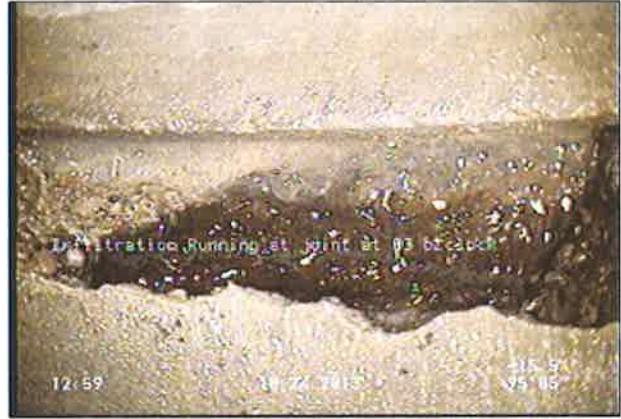
Photo: 10-11-18_10-10-6_6_24102013_130416_A.JPG Infiltration Running at joint at 03 o'clock
