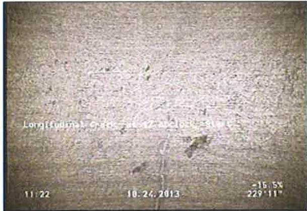
Photo: 10-9_10-10-6_19_24102013_112710_A.JPG Longitudinal Crack, at 12 o'clock, Start
