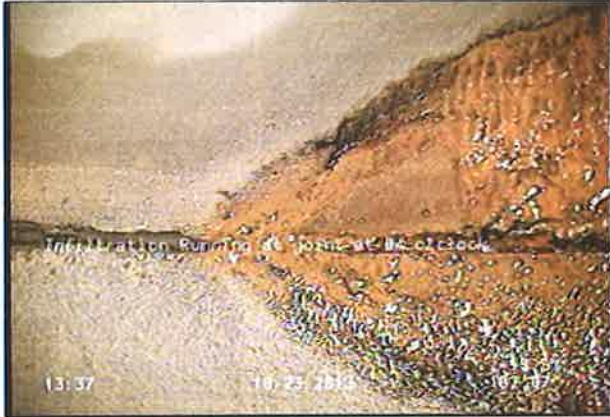
Photo: 10-7_10-8-21_6_23102013_134244_A.JPG infiltration Running at joint at 04 o'clock
