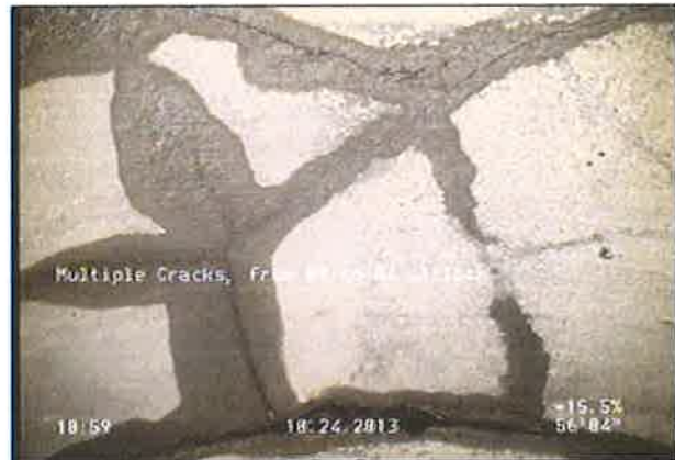
Photo: 10-9_10-10-6_6_24102013_110443_A.JPG Multiple Cracks, from 09 to 04 o'clock
