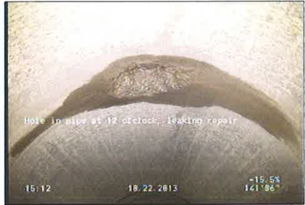
Photo: 2-16_MH-3_20_22102013_151719_B.JPG Hole in pipe at 12 o'clock / leaking repair
