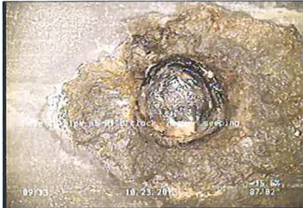
Photo: 10-3_10-4_12_23102013_091859_A.JPG Hole in pipe at 01 o'clock / repair seeping
