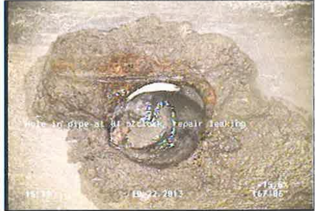
Photo: 2-16_MH-3_26_22102013_152412_A.JPG Hole in pipe at 01 o'clock / repair leaking
