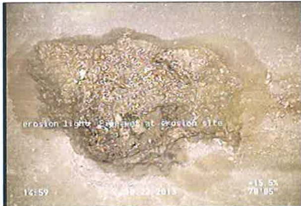
Photo: 2-16_MH-3_9_22102013_150452_A.JPG erosion light / Pipe wet at erosion site
