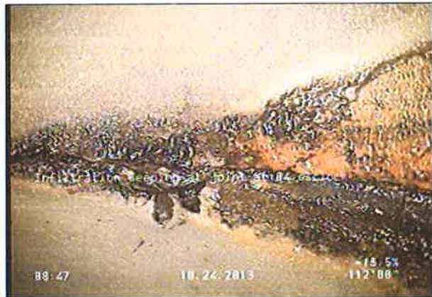
Photo: 10-8-21_10-9_5_24102013_085252_A.JPG Infiltration Seeping at joint at 04 o'clock
