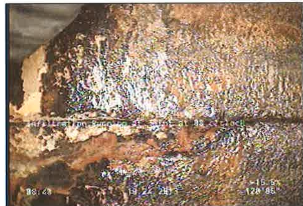
Photo: 10-8-21_10-9_6_24102013_085404_A.JPG Infiltration Running at joint at 08 o'clock
