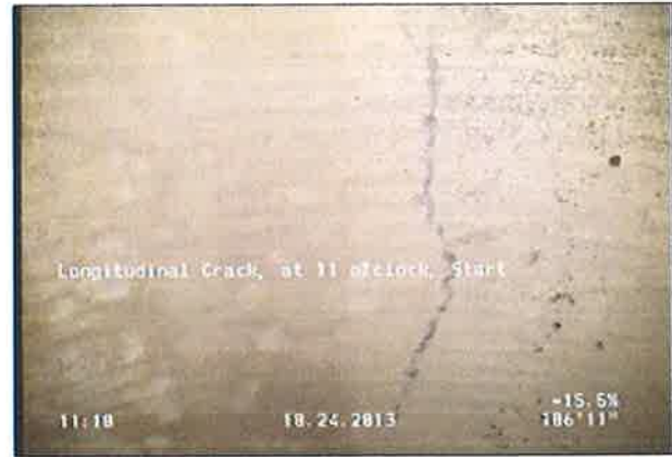
Photo: 10-9_10-10-6_12_24102013_111516_A.JPG Longitudinal Crack, at 11 o'clock, Start
