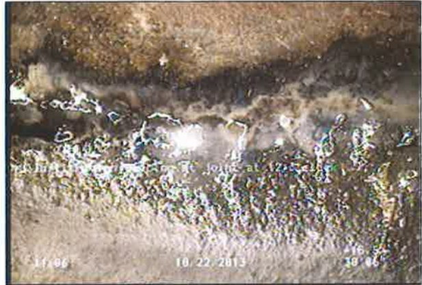
Photo: MH-1_2-16_4_22102013_111149_A.JPG Infiltration Seeping at joint at 12 o'clock
