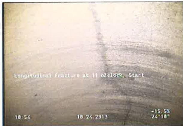
Photo: 10-9_10-10-6_2_24102013_105910_A.JPG Longitudinal Fracture at 11 o'clock, Start
