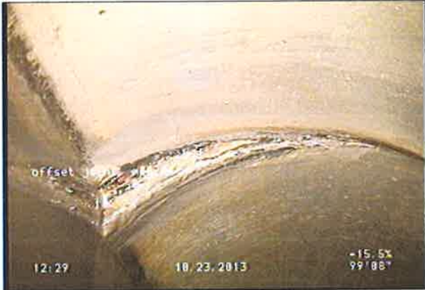
Photo: 10-5-7_10-7-21_10_23102013_123411_A.JPG offset joint, medium
