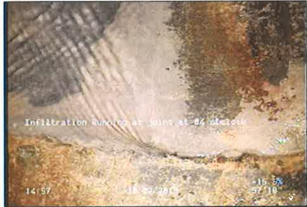
Photo: 2-16_MH-3_7_22102013_150240_A.JPG Infiltration Running at joint at 04 o'clock
