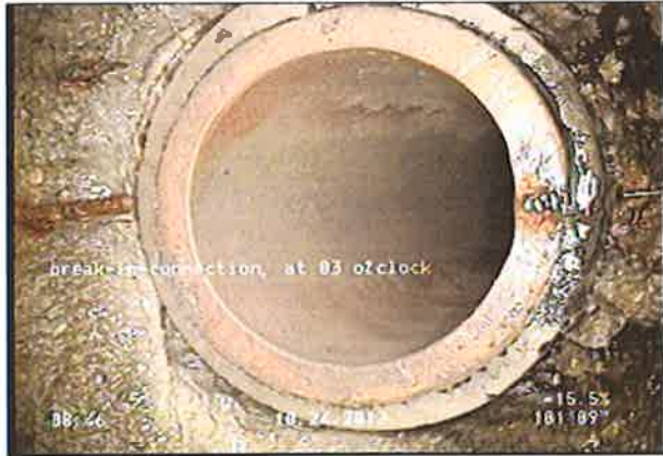
Photo: 10-8-21_10-9_4_24102013_085111_A.JPG break-in-connection, at 03 o'clock
