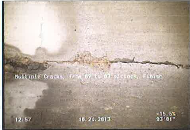
Photo: 10-11-18_10-10-6_5_24102013_130236_A.JPG Multiple Cracks, from 09 to 03 o'clock, Finish
