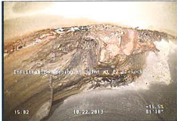
Photo: 2-16_MH-3_11_22102013_150715_A.JPG Infiltration Seeping at joint at 12 o'clock
