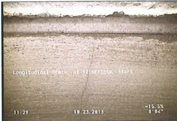
Photo: 10-6_10-5-7_2_23102013_113458_A.JPG Longitudinal Crack, at 12 o'clock, Start
