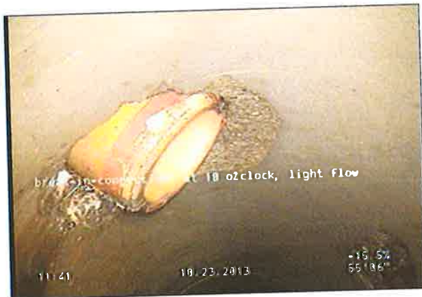
Photo: 10-6_10-5-7_5_23102013_114639_B.JPG break-in-connection, at 10 o'clock / light flow
