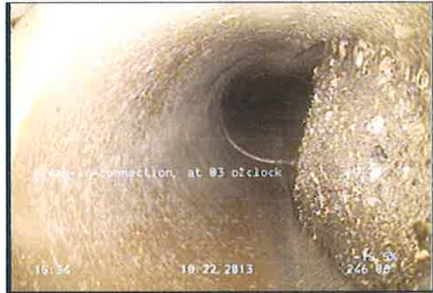
Photo: 2-16_MH-3_40_22102013_153951_A.JPG break-in-connection, at 03 o'clock
