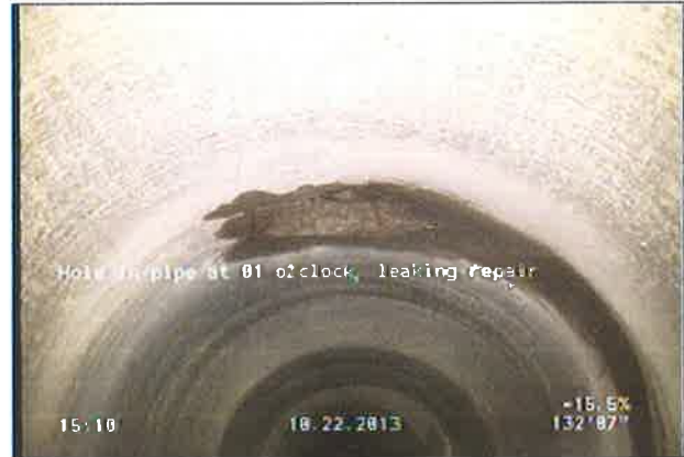
Photo: 2-16_MH-3_18_22102013_151530_B.JPG Hole in pipe at 01 o'clock / leaking repair
