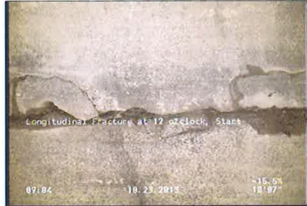
Photo: 10-3_10-4_5_23102013_090910_A.JPG Longitudinal Fracture at 12 o'clock, Start
