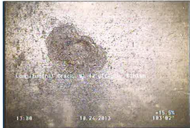
Photo: 10-11-18_10-10-6_8_24102013_130559_A.JPG Longitudinal Crack, at 12 o'clock, Finish
