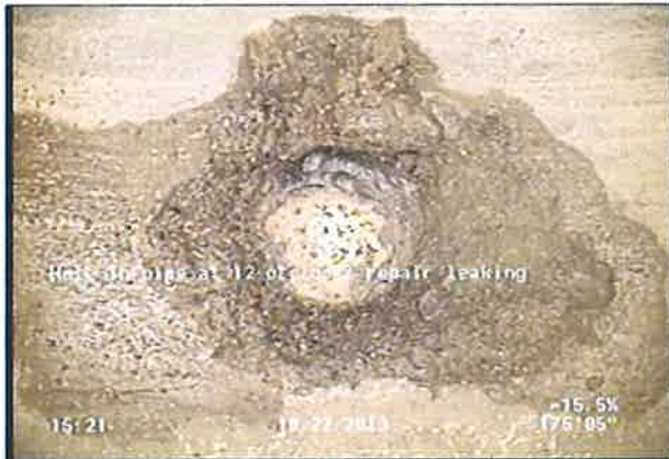
Photo: 2-16_MH-3_28_22102013_152620_A.JPG Hole in pipe at 12 o'clock / repair leaking
