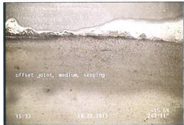
Photo: 2-16_MH-3_39_22102013_153833_A.JPG offset joint, medium / seeping
