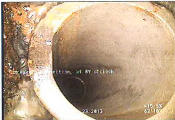
Photo: 10-7_10-8-21_3_23102013_133905_A.JPG break-in-connection, at 09 o'clock
