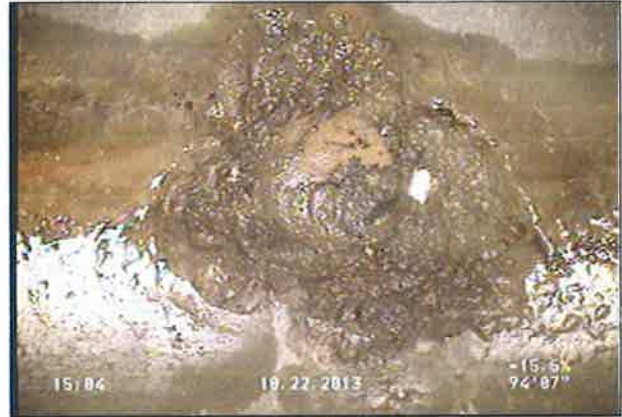
Photo: 2-16_MH-3_13_22102013_150929_A.JPG Hole in pipe at 12 o'clock / repaired but leaking
