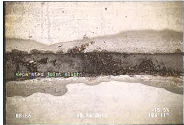
Photo: 10-8-21_10-9_9_24102013_090132_A.JPG separated joint slight
