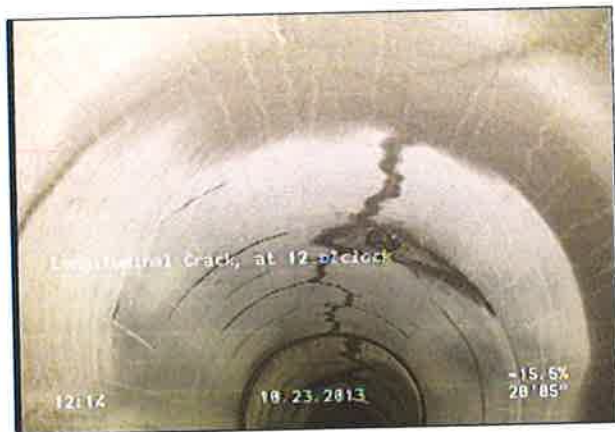
Photo: 10-5-7_10-7-21_3_23102013_121941_A.JPG Longitudinal Crack, at 12 o'clock, Start
