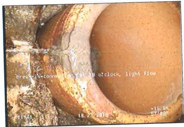
Photo: 10-6_10-5-7_5_23102013_114625_A.JPG break-in-connection, at 10 o'clock / light flow
