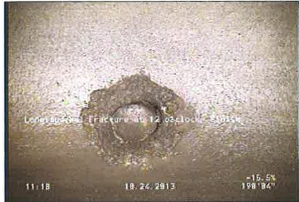
Photo: 10-9_10-10-6_17_24102013_112322_A.JPG Longitudinal Fracture at 12 o'clock, Finish
