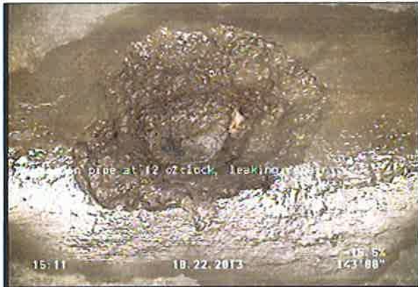
Photo: 2-16_MH-3_20_22102013_151705_A.JPG Hole in pipe at 12 o'clock / leaking repair
