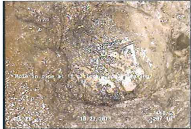
Photo: 2-16_MH-3_32_22102013_153138_A.JPG Hole in pipe at 11 o'clock / repair leaking
