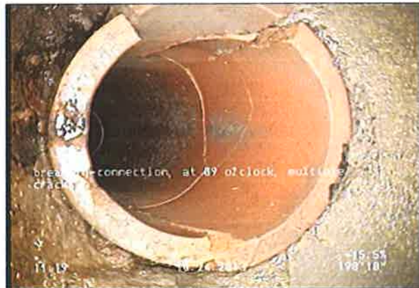
Photo: 10-9_10-10-6_18_24102013_112435_A.JPG break-in-connection, at 09 o'clock / multiple cracks
