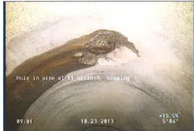
Photo: 10-3_10-4_2_23102013_090618_B.JPG Hole in pipe at 11 o'clock / seeping
