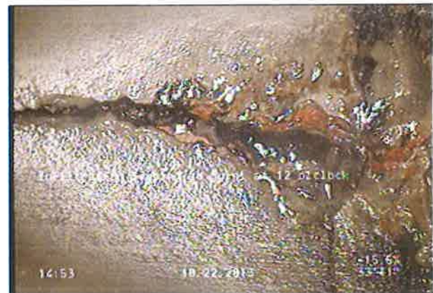
Photo: 2-16_MH-3_5_22102013_145907_A.JPG Infiltration Seeping at joint at 12 o'clock
