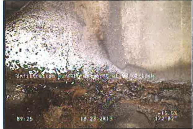
Photo: 10-3_10-4_18_23102013_093033_A.JPG Infiltration Running at joint at 08 o'clock
