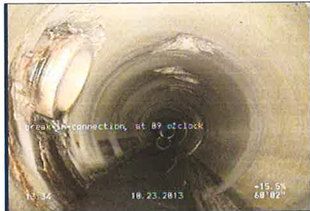
Photo: 10-7_10-8-21_3_23102013_133920_B.JPG break-in-connection, at 09 o'clock
