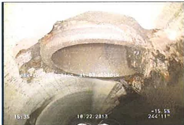
Photo: 2-16_MH-3_40_22102013_154011_B.JPG break-in-connection, at 03 o'clock
