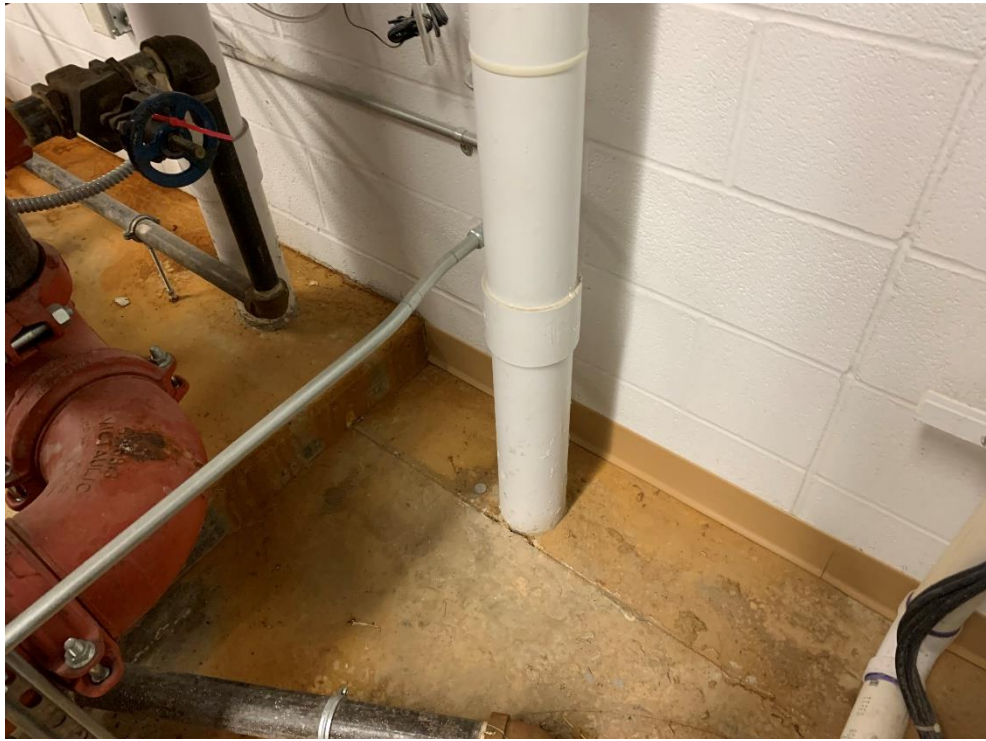
Photograph No. 5 – Sub-slab Depressurization System in basement, depicting stack discharge piping floor penetration.
