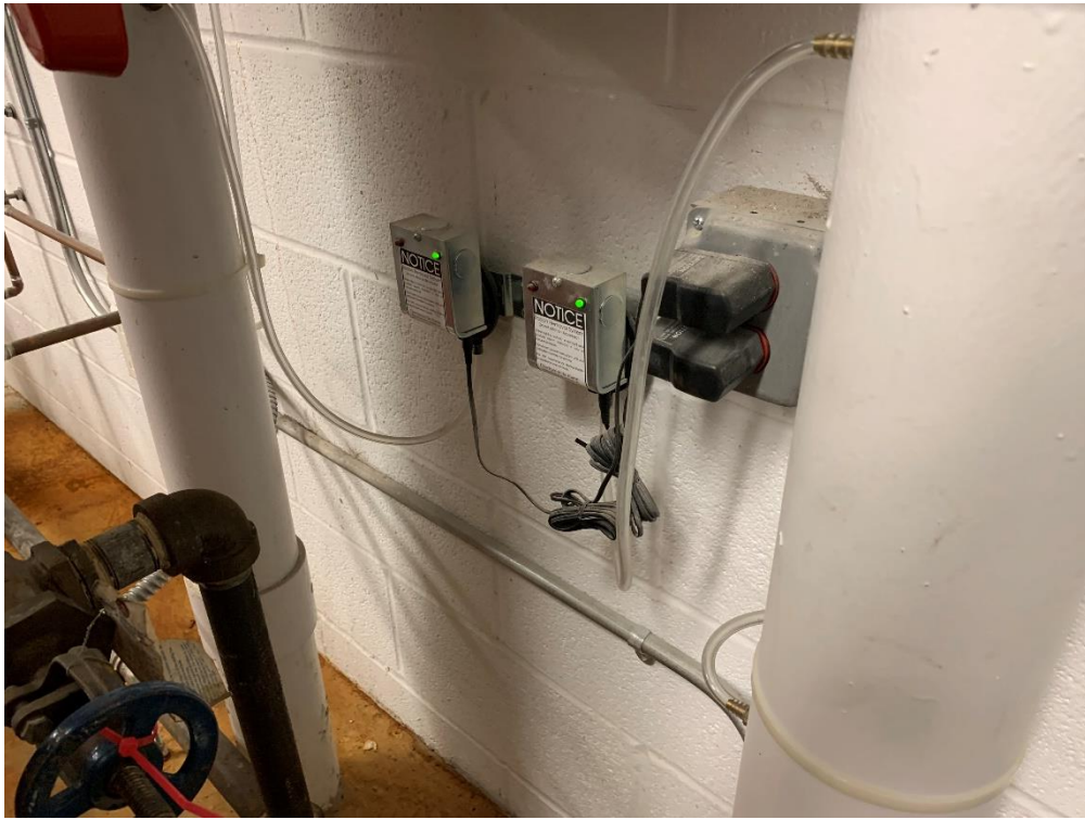
Photograph No. 3 – Sub-slab Depressurization System in basement, depicting alarms.
