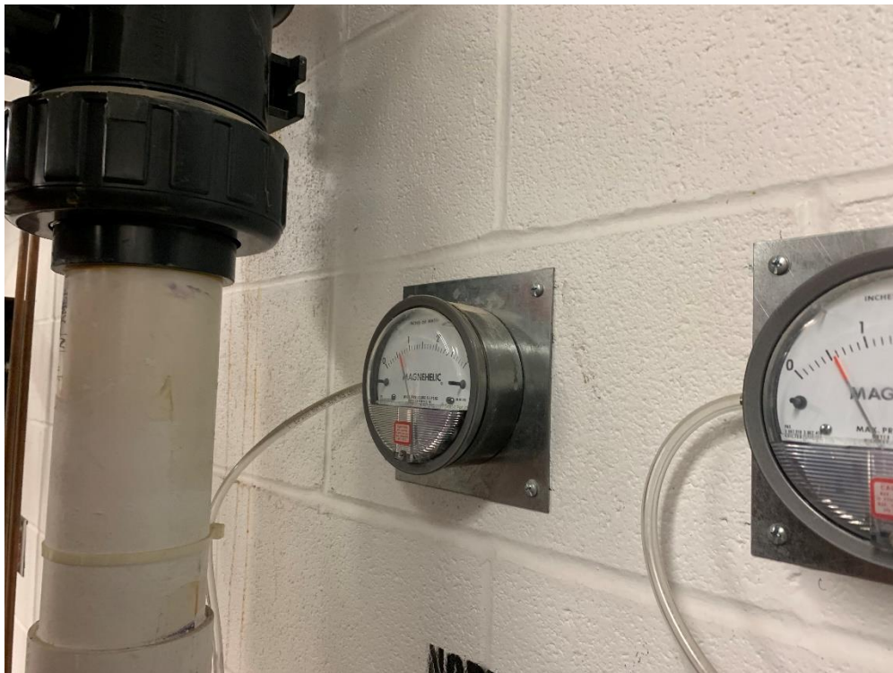
Photograph No. 2 – Sub-slab Depressurization System in basement, depicting pressure gauges.
