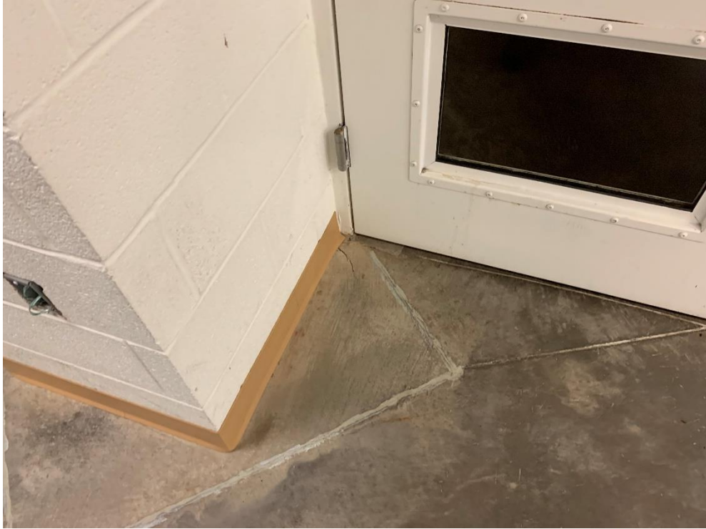
Photograph No. 6 – Minor crack in concrete floor in men's jail.
