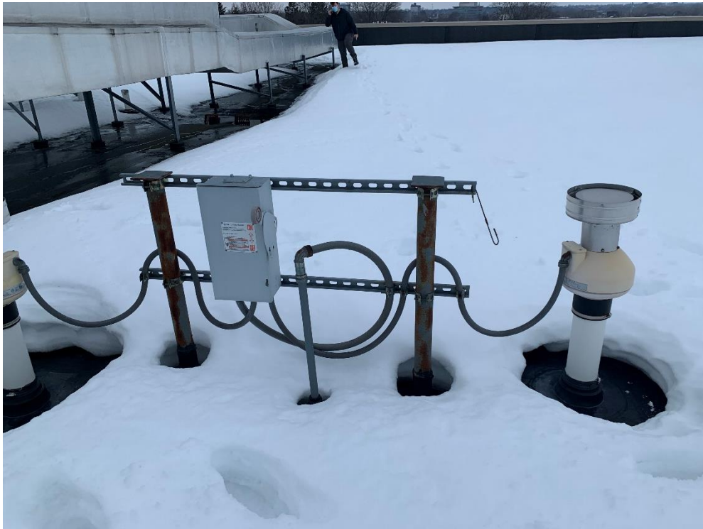
Photograph No. 7 – Sub-slab Depressurization System discharge vents and blowers and power control for discharge vents.
