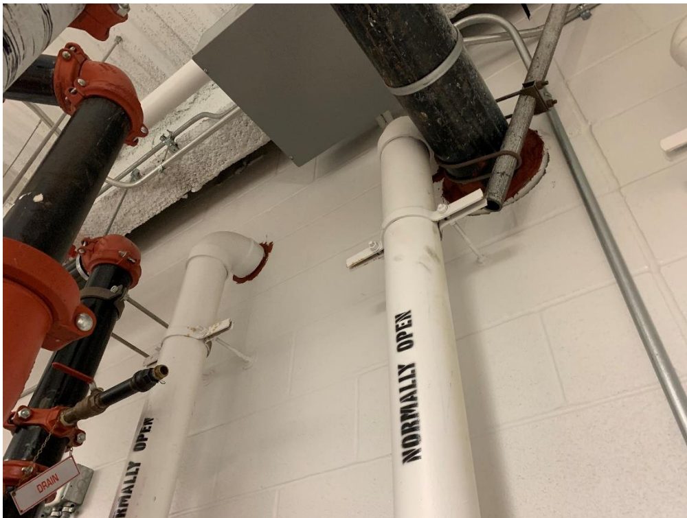
Photograph No. 4 – Sub-slab Depressurization System in basement, depicting stack discharge piping.
