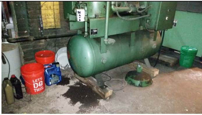
Leak near compressor in boiler room of Site Building 2
