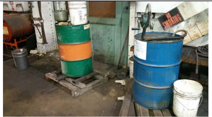
Drum storage/dispensing area in Machine Shop Main Floor portion of Site Building 2
