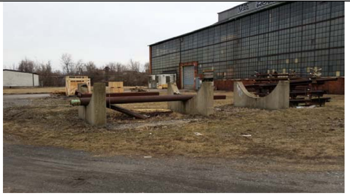
Concrete cradles and containment for removed 20,000-gallon AST west of Site Building 2
