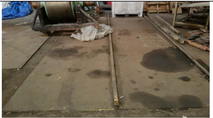
Covered pit in Fabricating Department portion of Site Building 2 used as storage
