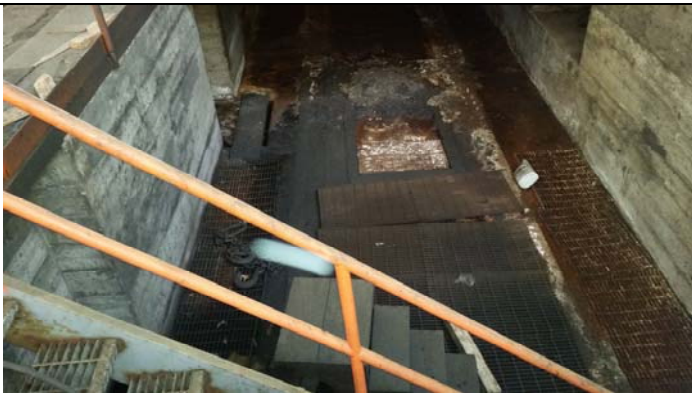
Open pit in Fabricating Department portion of Site Building 2 used as storage
