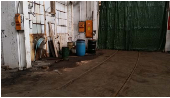
Drum area with staining at west end of Fabricating Department portion of Site Building 2
