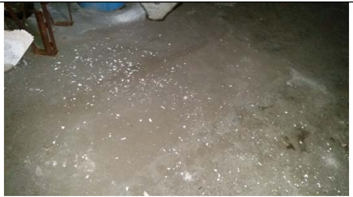
Concrete patch in locker room in Site Building 2 from closure of 10,000-gallon UST
