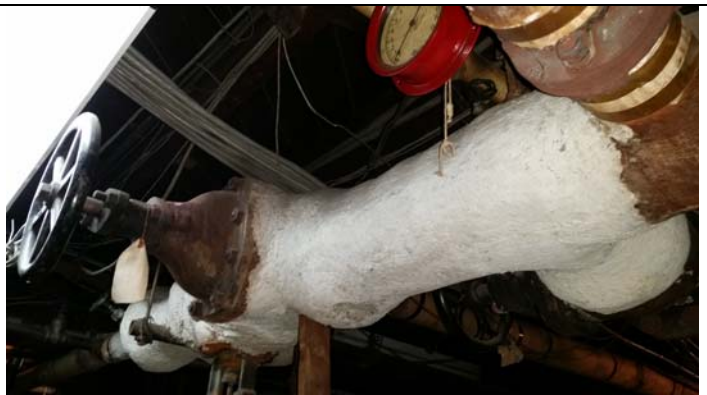
Suspected ACM in basement of Site Building 1
