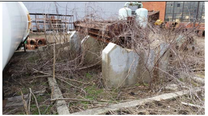
Concrete cradles and containment for AST east of Storage Building & Receiving portion of Site Building 2
