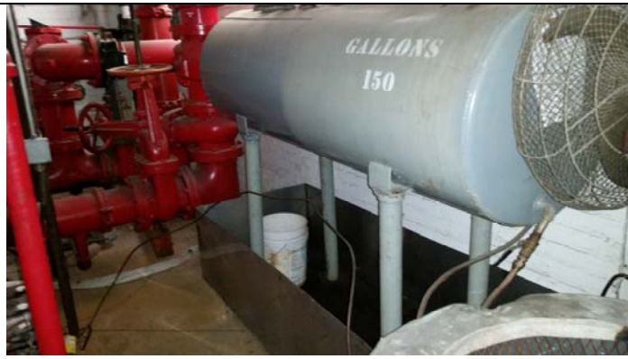
Fuel tank for fire protection system in Site Building 3
