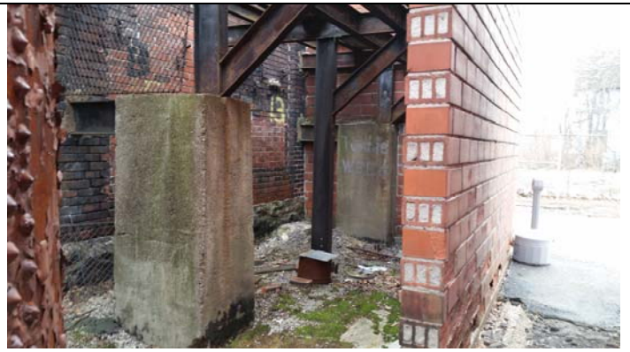
Former transformer location west of Site Building 2
