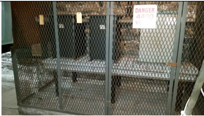
Transformers in basement of Site Building 1
