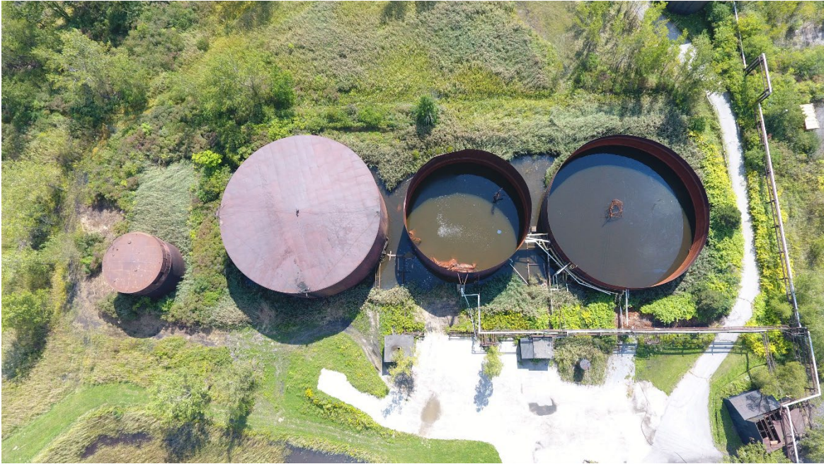
Photograph No. 1 ST24 to ST21 Tanks (Left to Right) Before Demolition (Note: The small black tank north (below in photograph) was ST20)
