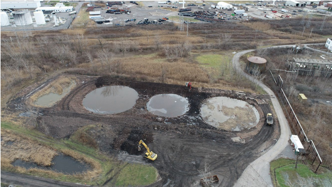
Photograph No. 2 Former Location of ST24 to ST21 (Left to Right) After Removal of the Tanks (Before Dewatering)
