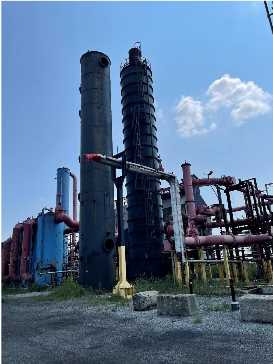
Photograph No. 3 West Flare Piping
