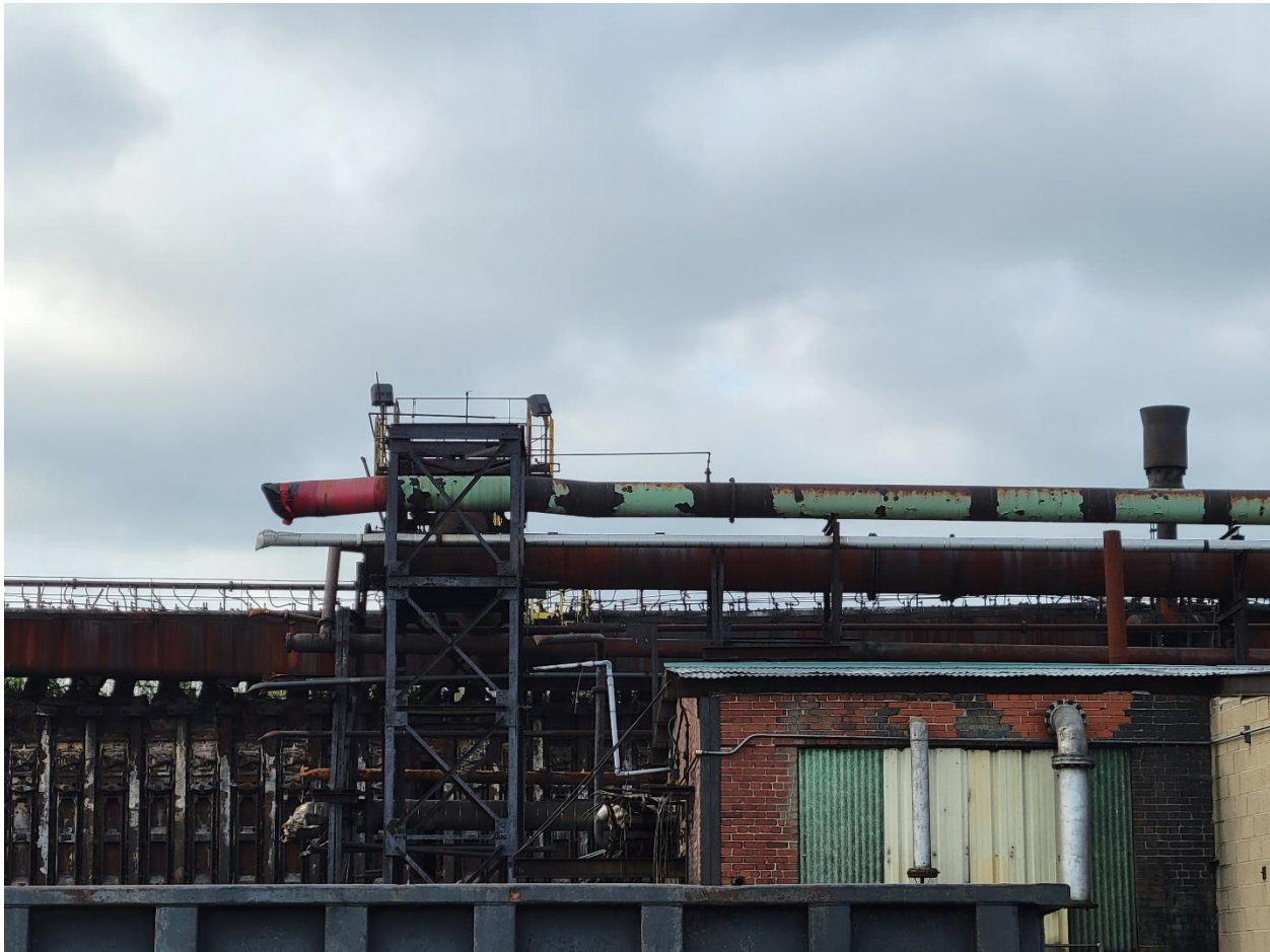
Photograph No. 5 COG Pipe at Pump House Looking South
