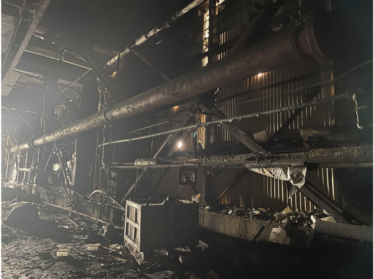
Photograph D 8: Taken to illustrate surrounding piping.
