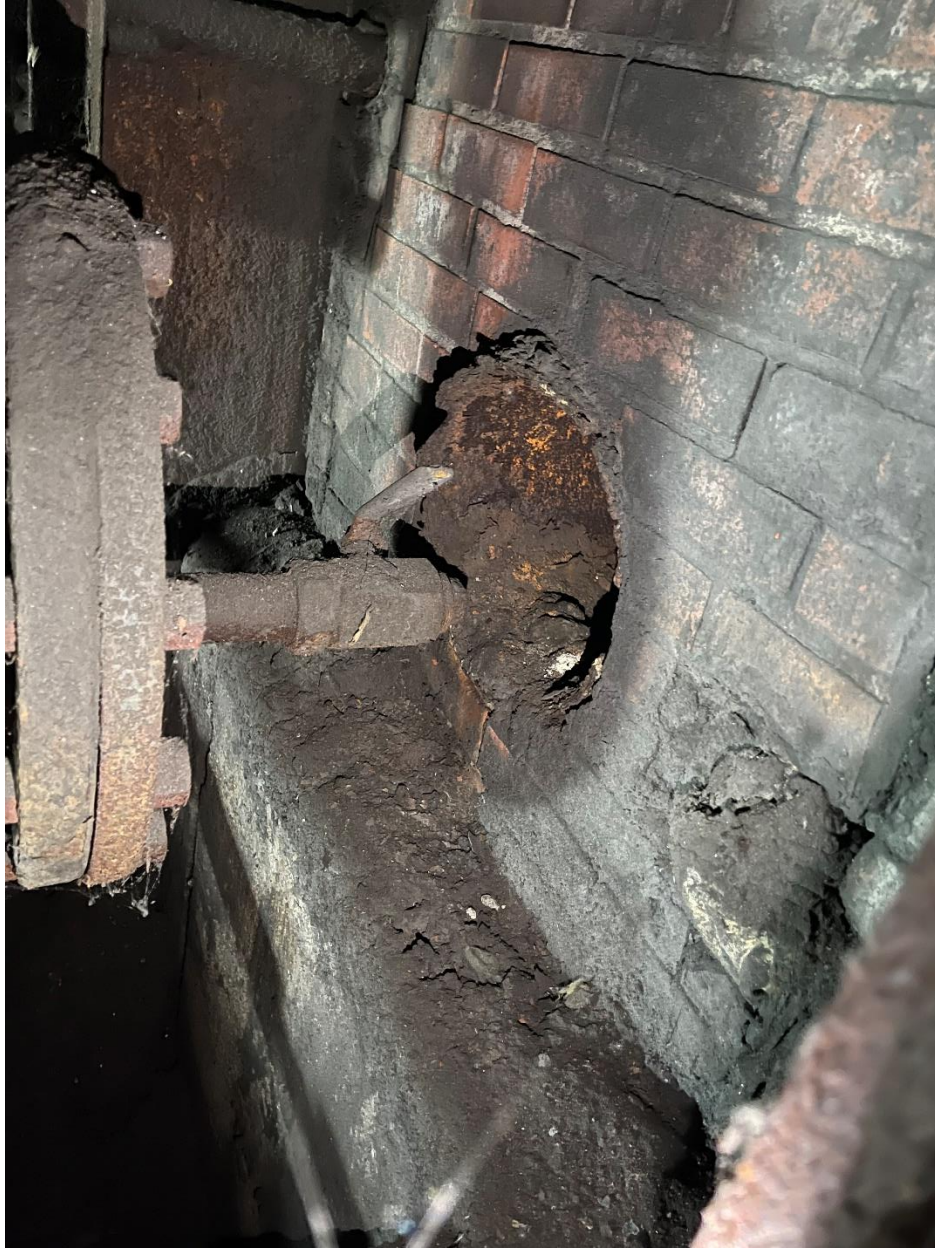
Photograph D 7: The bolted flange is the end of the COG line it is capped at this hole.
