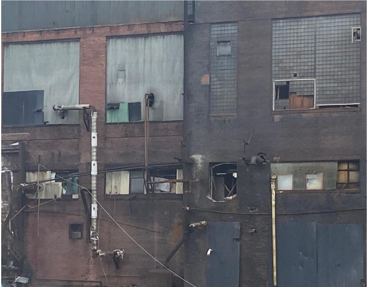
Photograph No. 6 COG Pipe Penetrating the South Boiler House Wall (Looking North)
