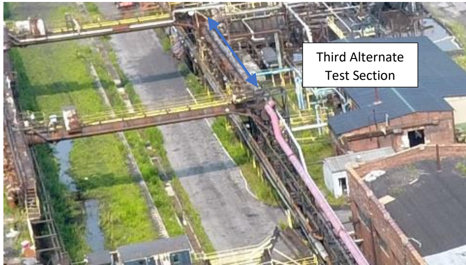
Photograph No. 4 Location of COG Pipe Between the Crossover Pipes (All COG Pipe East of the Crossover Pipe has been removed)
