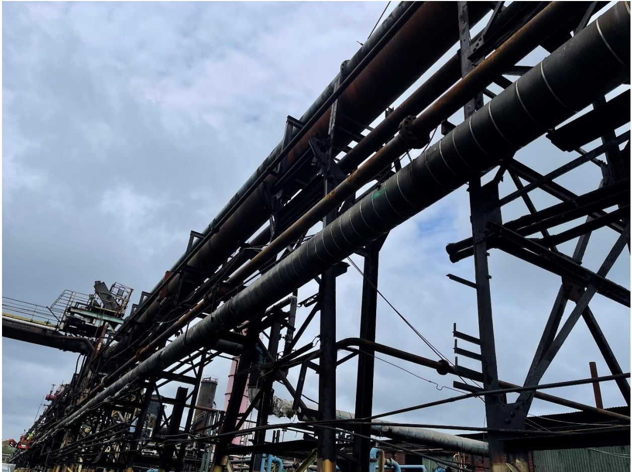
Photograph D 2: Section of pipe rack evaluated. Note west crossover pipe on left side of image.
