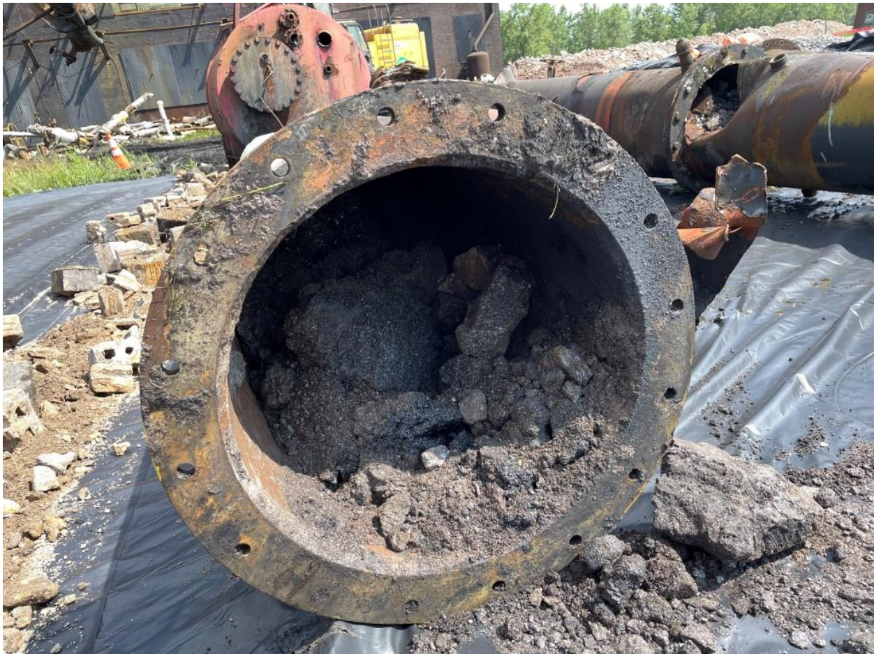
Photograph No. 1 Coke Oven Gas Pipe and Residual
