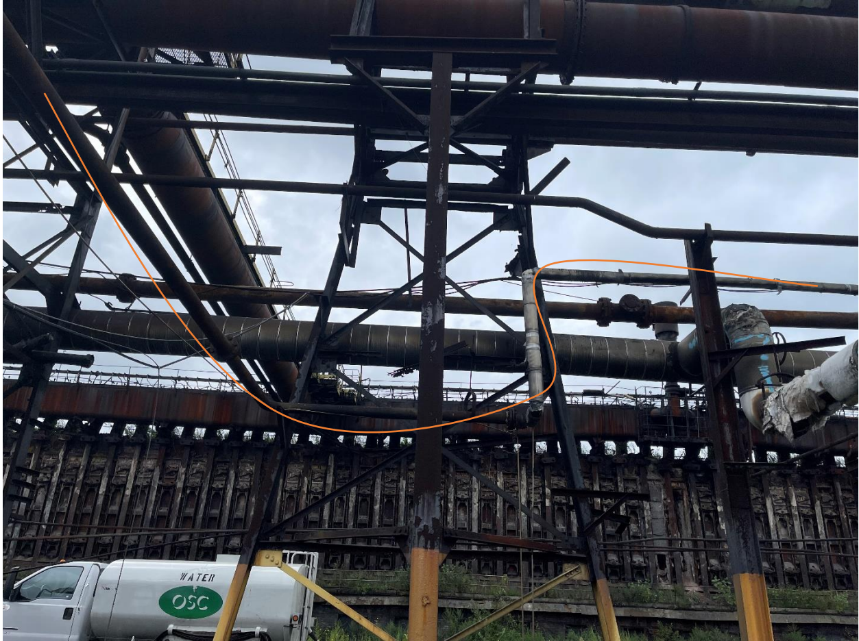
Photograph D 4: Pipe 11 out of 12. It comes from the Pump House and continues down the rack.
