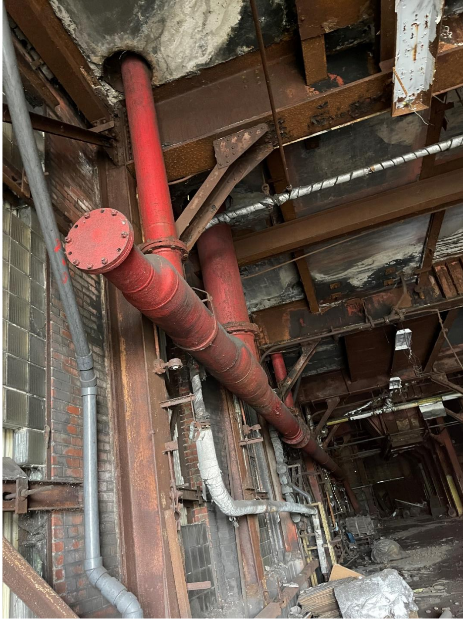
Photograph D 6: The COG line inside the Boiler House is approximately 92ft in length.
