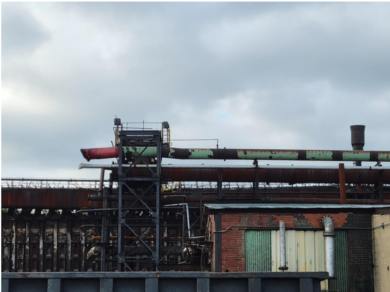
Photograph D 1: Pipe rack supporting the east crossover pipe to Battery.
