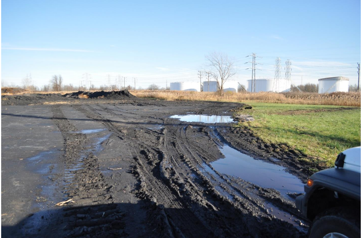
Photograph No. 6 Bend in South Ditch Road Pavement Intermittently Degraded or Missing.
