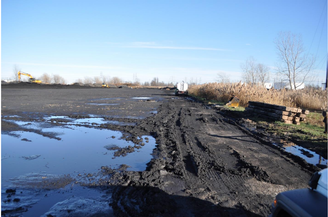
Photograph No. 3 Accumulations of Water Rising to potentially Flow Around Check Dams at CB-03
