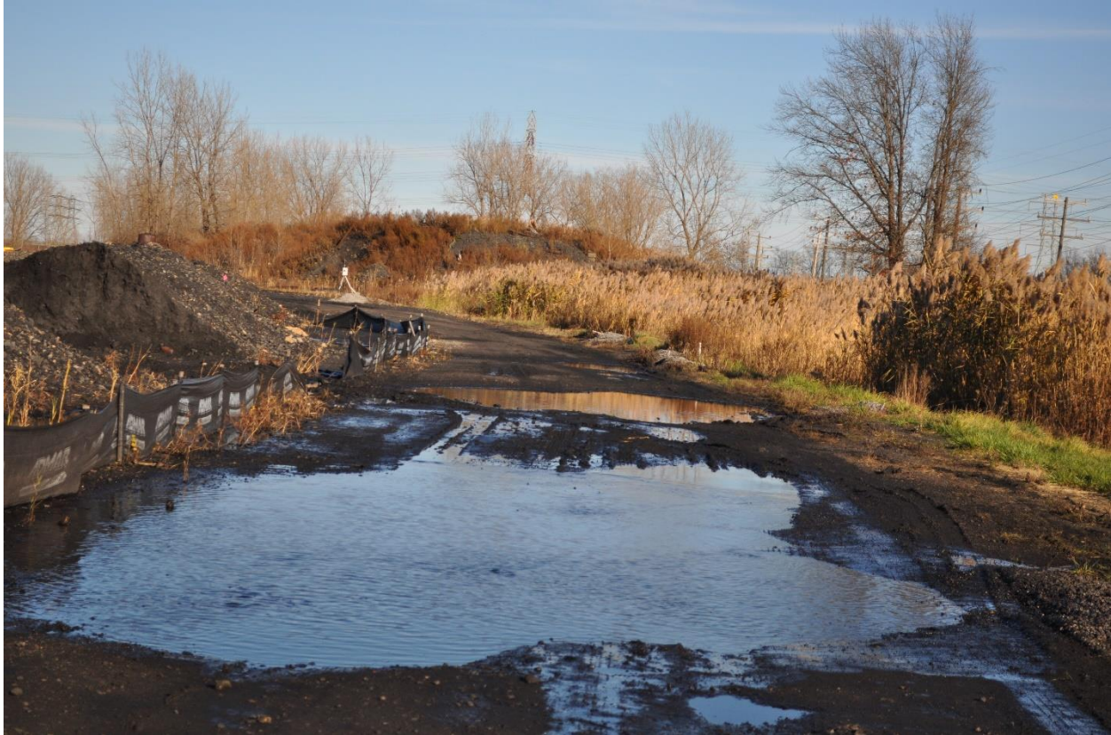
Photograph No. 8 East End of South Ditch Road Pavement Missing until Point Near Air Monitoring Station
