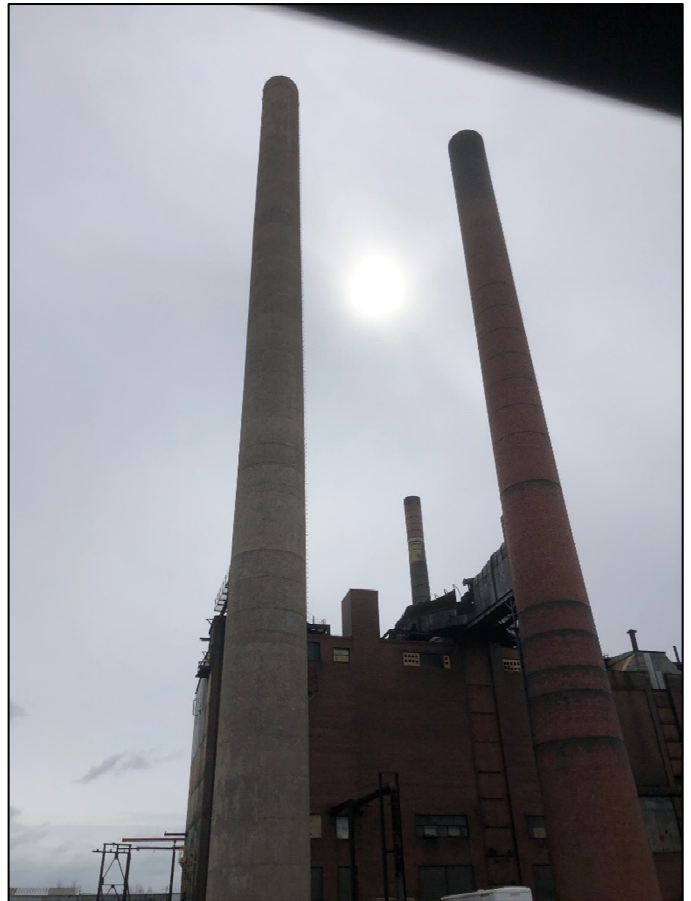
The two boiler house stacks (foreground) and the top of the waste heat stack (center-back), looking south. All three stacks will be demolished during Summer 2021 (March 2021).
