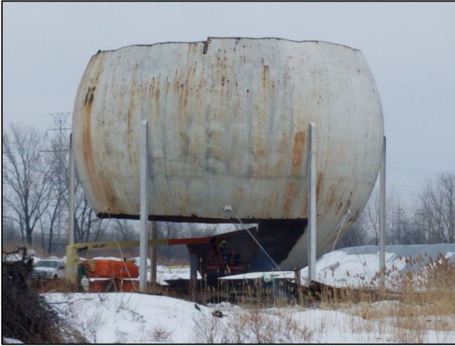
Demolition of the gas holder that was used to store excess coke oven gas prior to use in the coking process or being sold for off-site use (February 2021).
