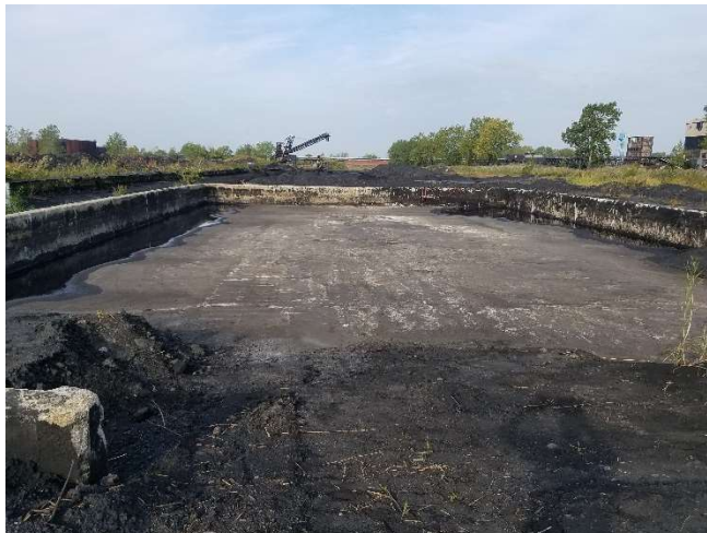
The 'Mixing Pad' after stormwater was pumped out and treated. Sampling to determine the extent of impacts from past operations is ongoing. All materials are being properly characterized for decontamination or off-site disposal (DEC photo).
