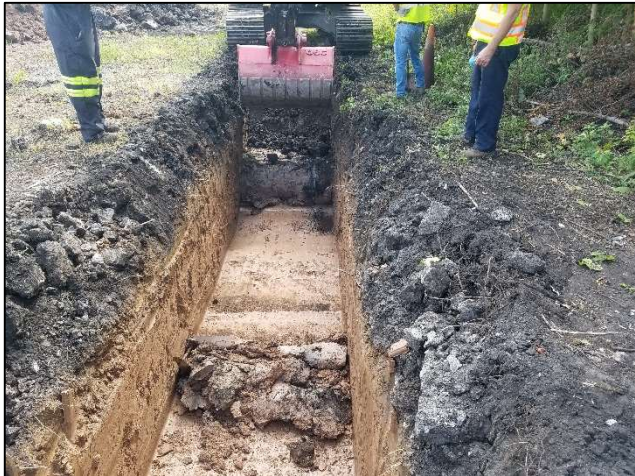
Test pit to investigate soil surrounding former water supply pipe (DEC photo) under the Abandoned Pipeline IRM.
