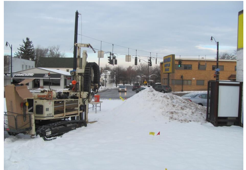
6. Location of BH-2 facing west at corner of Main and Hertel Ave.
