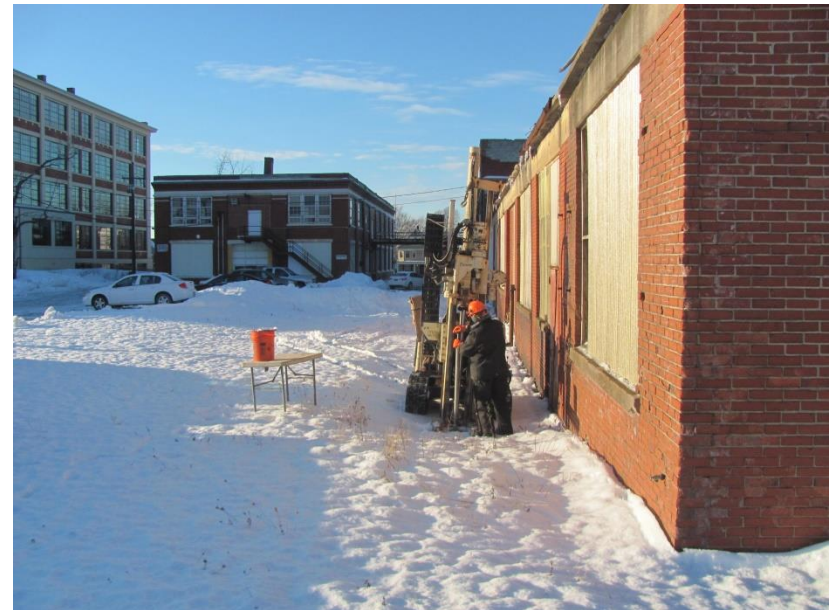
44. Location of Borehole BH-16 adjacent to west side of Building 4 facing north-northwest
