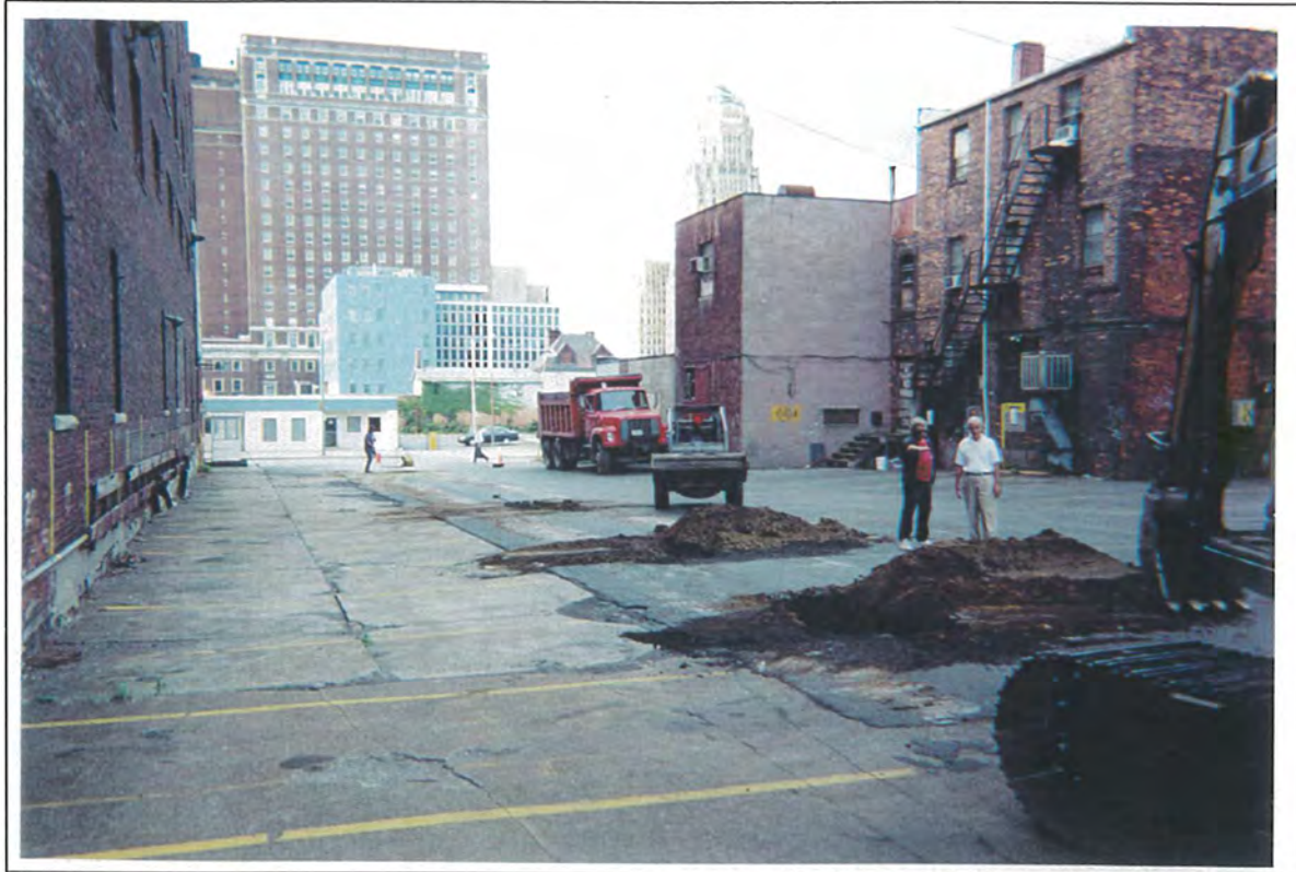
Photo 03: Test pits TP-6 (foreground), TP-5 and TP-4 locations and typical soil/fill lithology.
