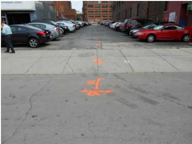
Underground utilities were marked on the property before the start of soil sampling work
