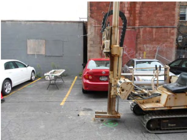
Soil boring GP-7 is located on the west side of the parking lot near Building #2
