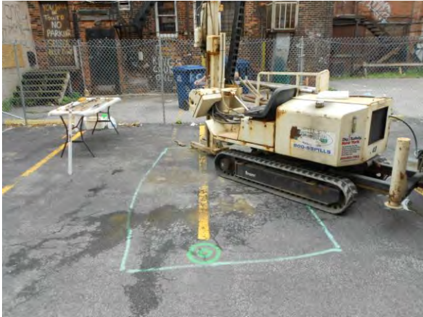
Soil boring GP-5 is located on the west side of the parking lot near Building #3
