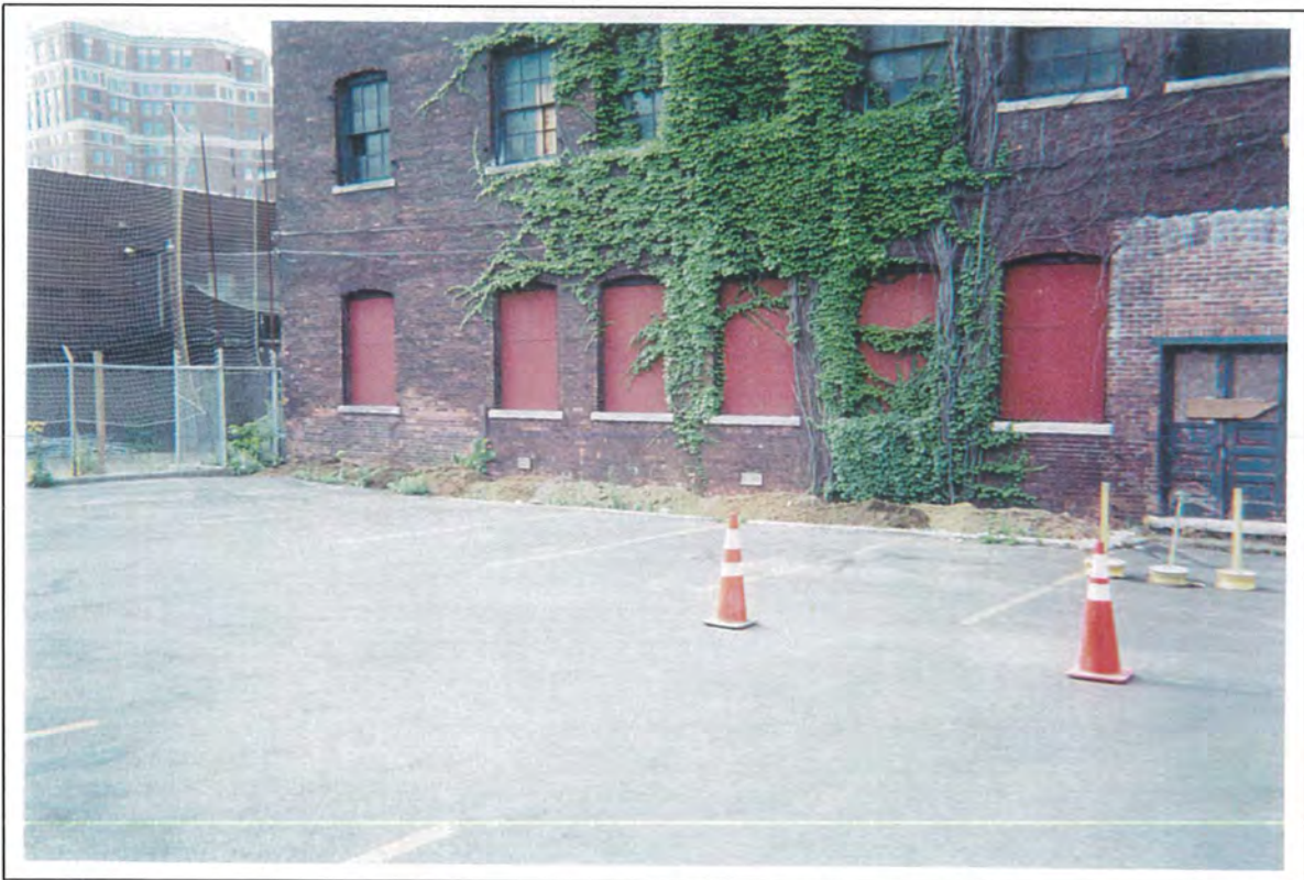
Photo 06: North end of parking garage showing staging area for excess excavation material.
