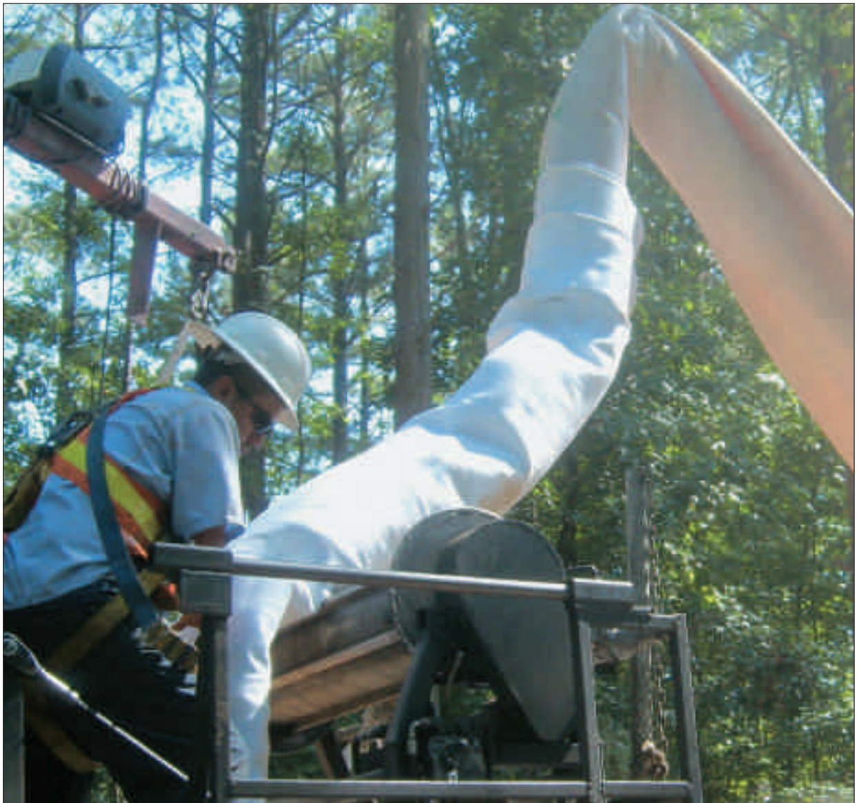
Lanzo Lining Services crew preparing liner for direct inversion installation of CIPP
