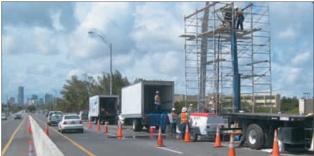
Trenchless CIPP rehabilitation of a pipe running under a busy highway during rush hour traffic
