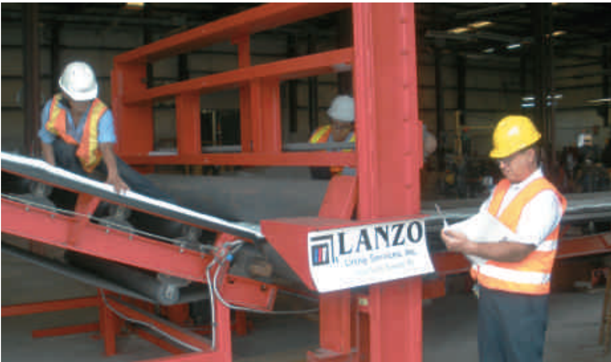
Quality controlled tube impregnation at one of Lanzo Lining Services' state of the art wet out facilities
