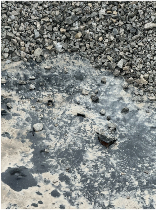
Photo 1 : Additional damage to geomembrane
