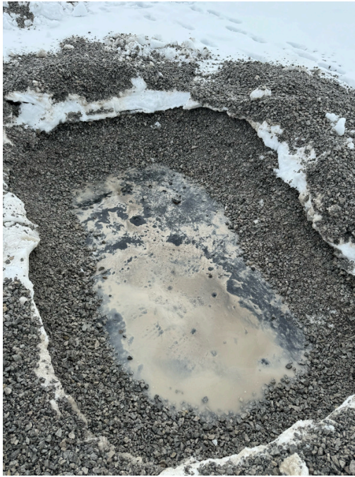
Photo 7 : Completed gravel removal with additional damage
