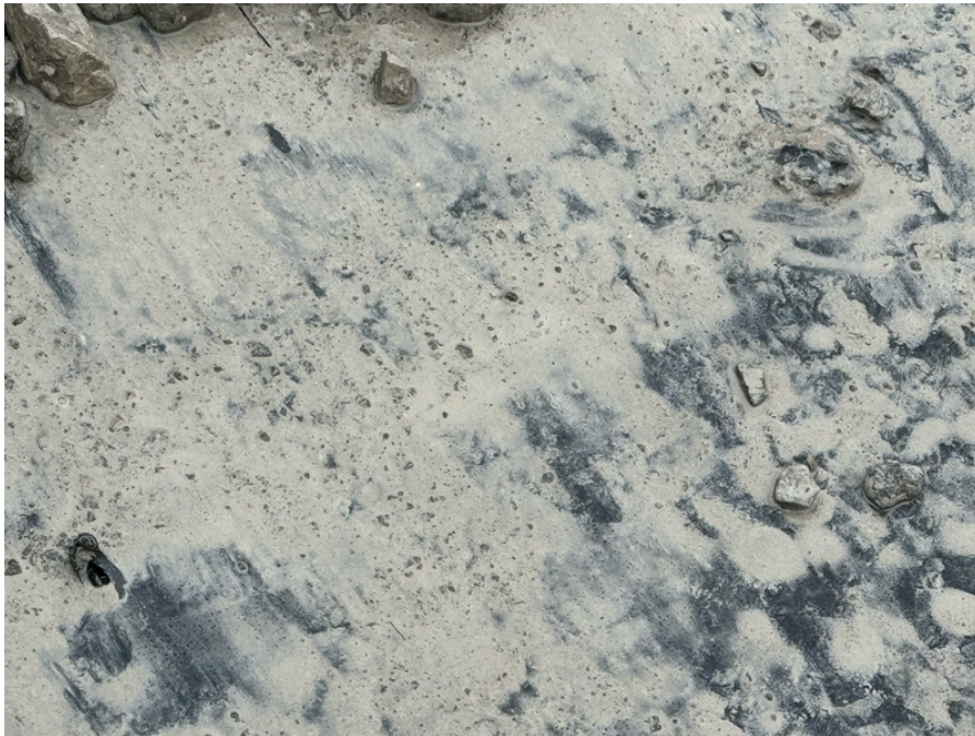
Photo 2 : Additional geomembrane damage
