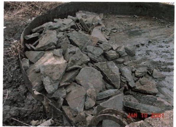
Revealing that the bottom of the tank had been filled with a layer of concrete for an undetermined reason.
