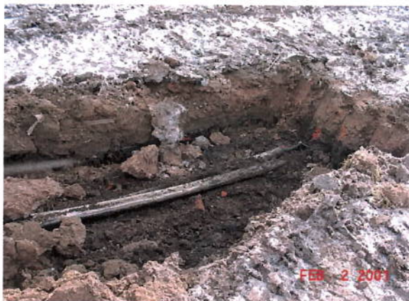
Product delivery lines are also still on site.
