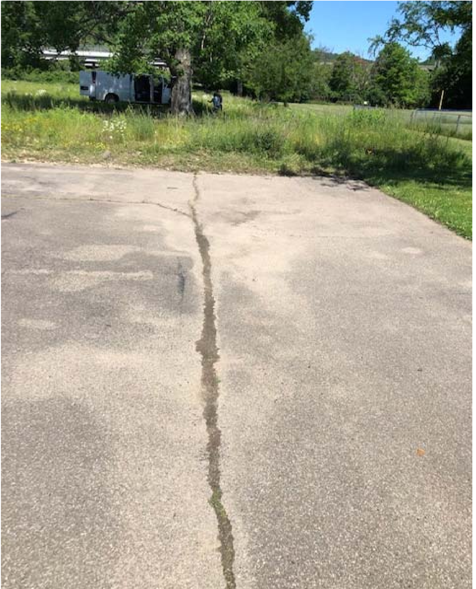
View of repaired asphalt cover located on the eastern portion of the Employee Parking Lot, facing northwest. View of groundwater monitoring event at monitoring well MW-E, amid the soil/vegetative cover and mulch cover (below visible tree) at top of photo.
