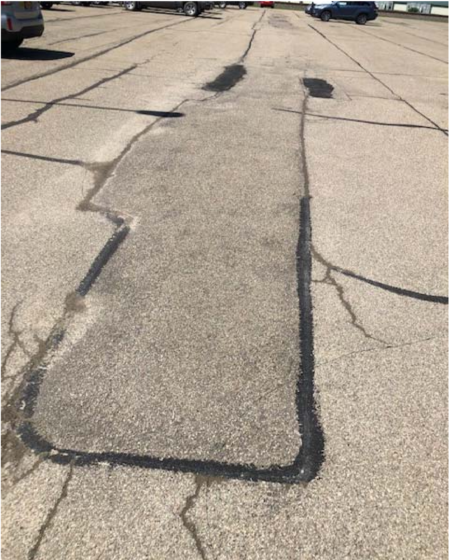
Typical view of the asphalt repairs completed on the western portion of the Employee Parking Lot, facing west.
