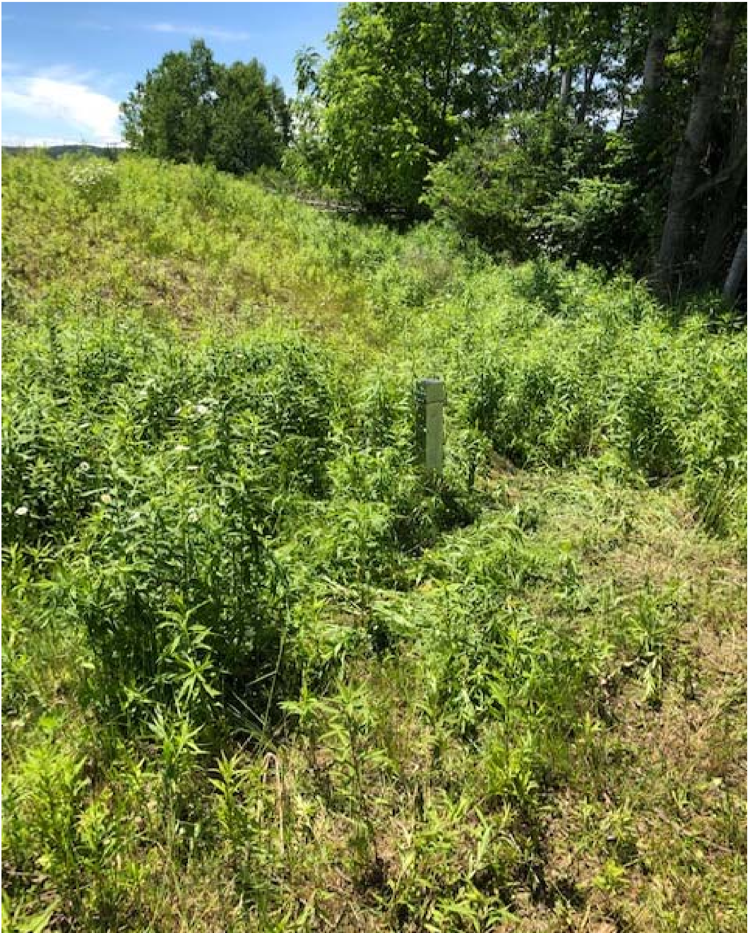
Typical view of a monitoring well protective casing, located on the northern portion of the Site, facing south.
