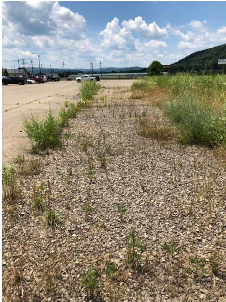
Typical view of drainage channel, located adjacent to the north of the Employee Parking Lot, facing west.
