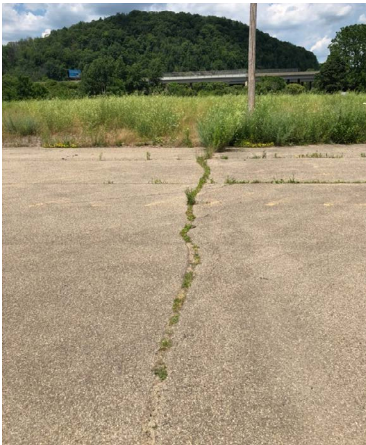
Typical view of vegetation growing in cracks in the asphalt cover, facing north.
