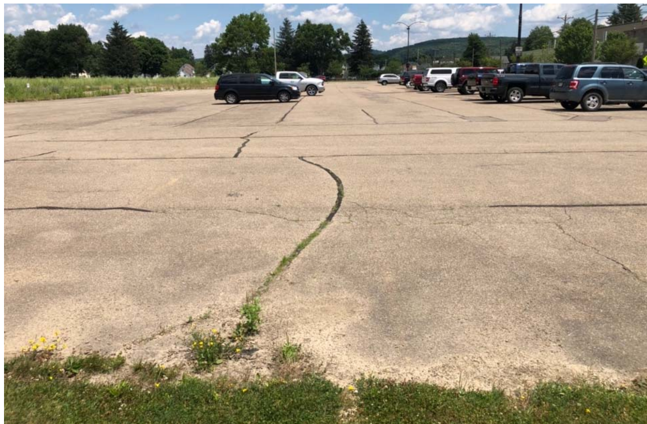
Western portion of the asphalt cover over the Employee Parking Lot, located on the southern portion of the Site, facing east.
