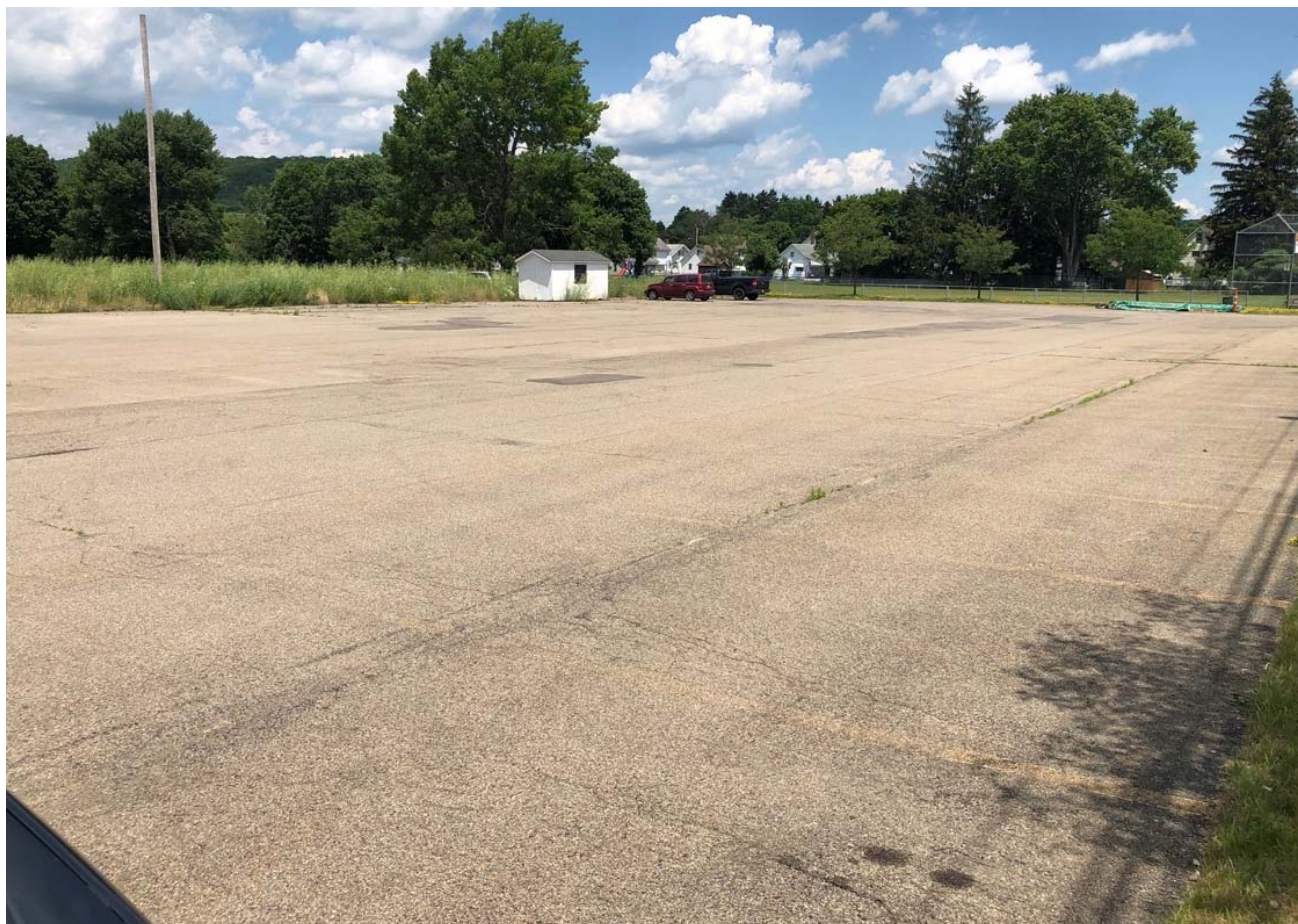
Eastern portion of the asphalt cover over the Employee Parking Lot, located on the southern portion of the site, facing northeast.
