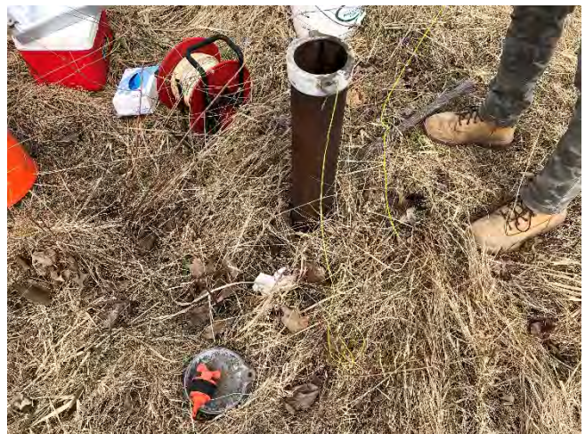
Photo No. 12 OW-3 missing lock
