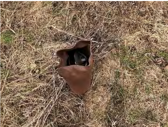
Photo No. 5 Unknown Well (north of IW-14) casing damaged
