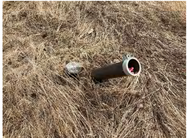
Photo No. 16 Unknown well destroyed
