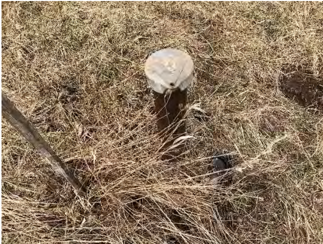
Photo No. 13 OW-2 missing lock
