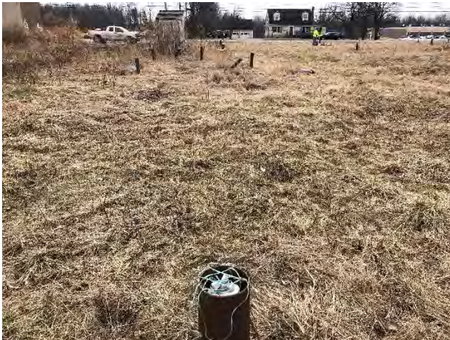
Photo No. 15 IW-4 cover broken off
