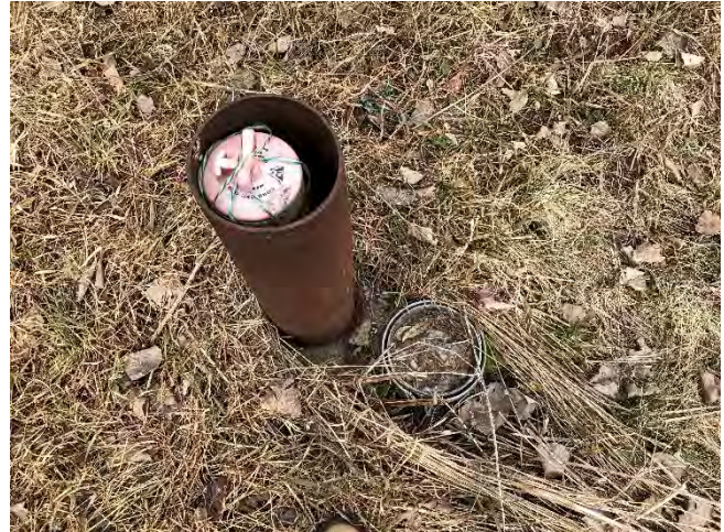
Photo No. 4 IW-14 cover broken off
