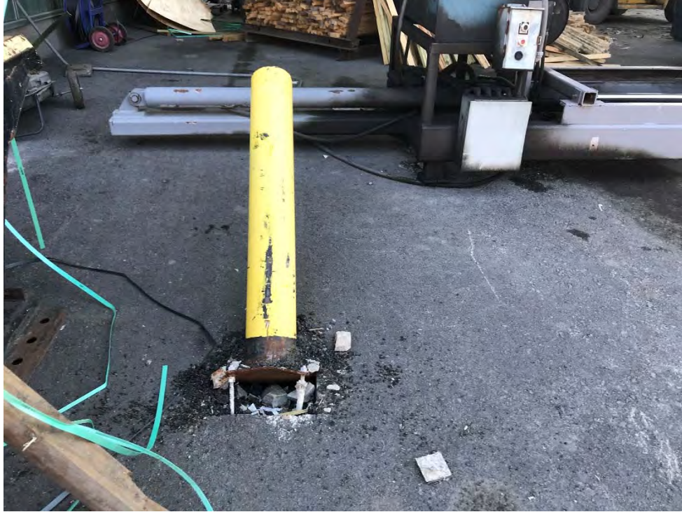
Photograph 17: Damaged bollard along southwest perimeter of the treatment process building. Localized damage is not considered a risk to onsite workers or the environment.
