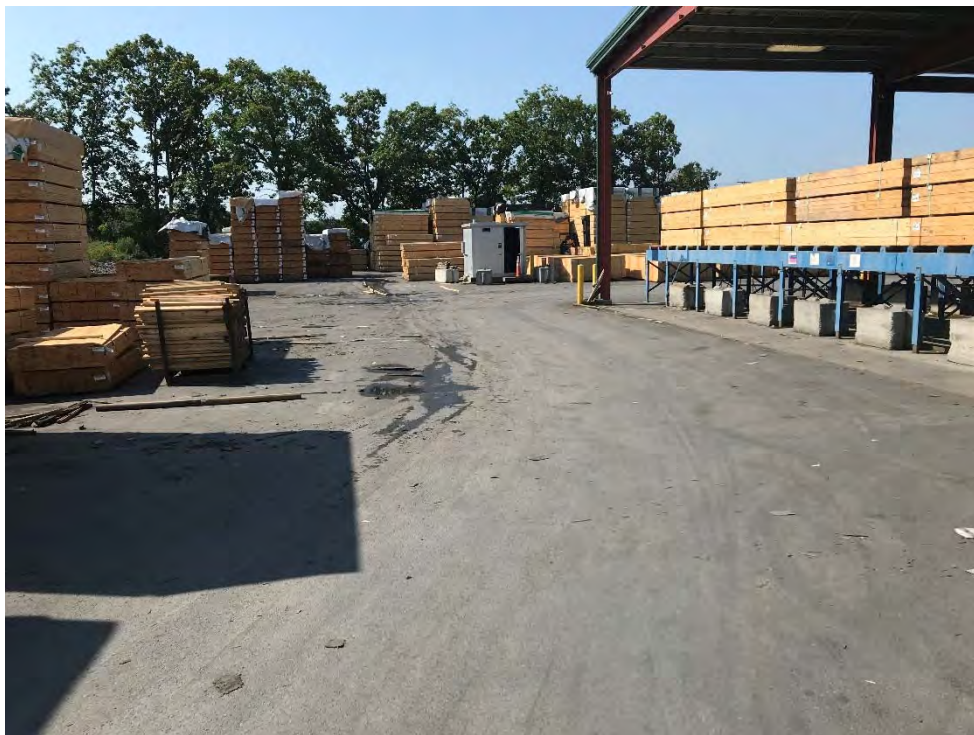
Photograph 16: Southern portion of protective asphalt cover in acceptable condition directly east of the treatment process building. Looking south.
