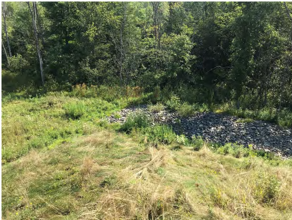
Photograph 6: Southern abatement berm and perimeter drainage with soil cover in acceptable condition. Looking northeast.
