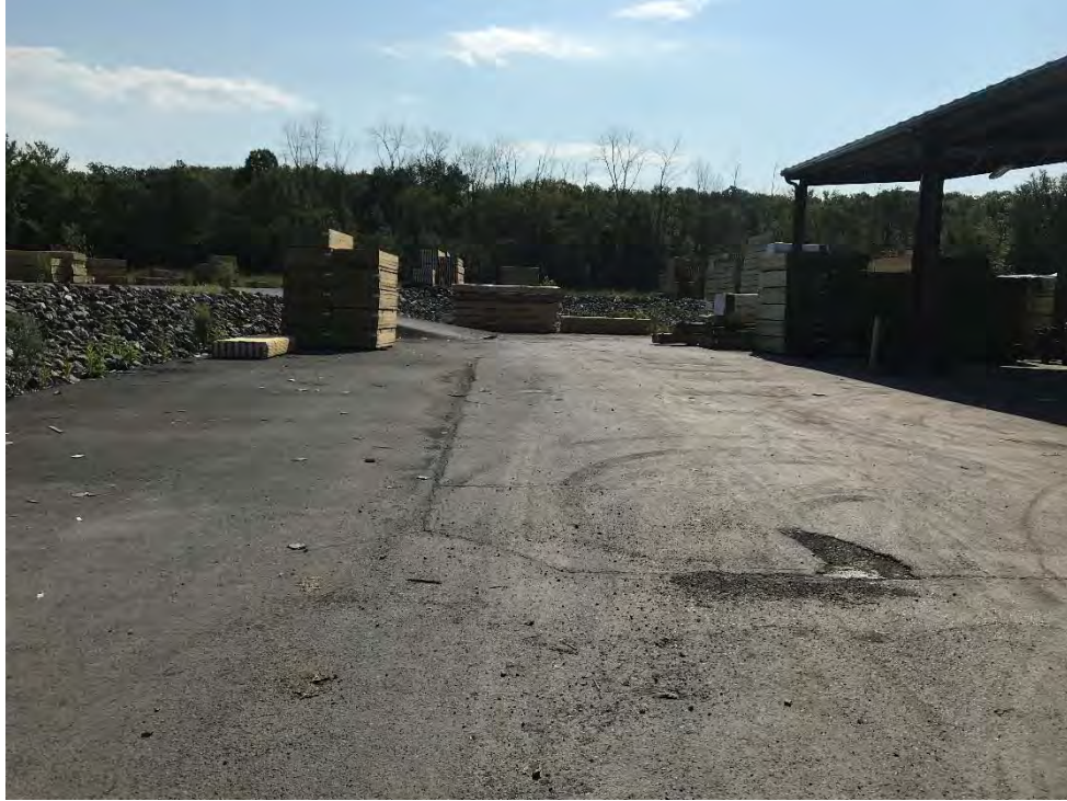
Photograph 15: Central portion of protective asphalt cover in acceptable condition directly north of the treatment process building. Looking east.
