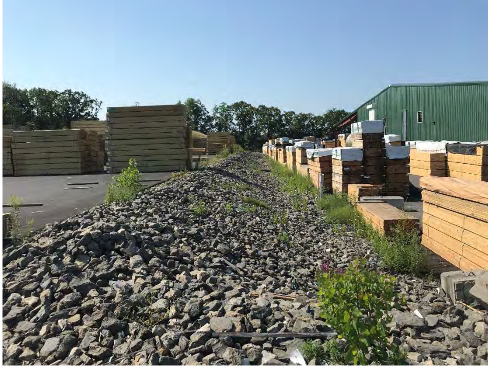
Photograph 9: Grade transition area between treatment process building and storage area in acceptable condition. Looking south.
