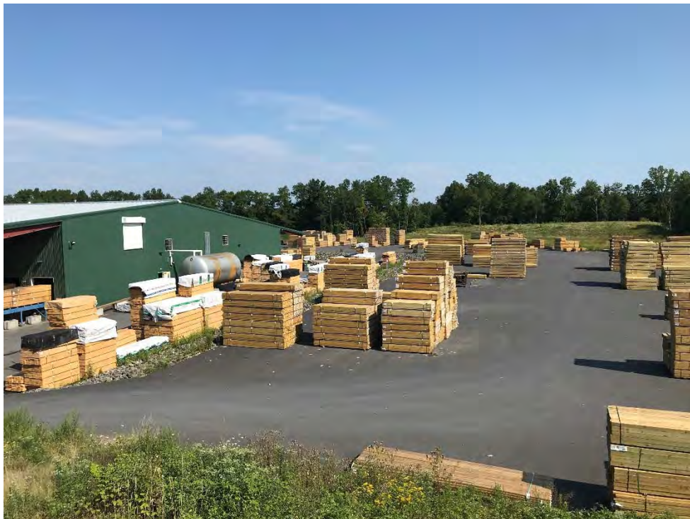
Photograph 2: Overview of central portion of protective asphalt cover in acceptable condition. Looking north.
