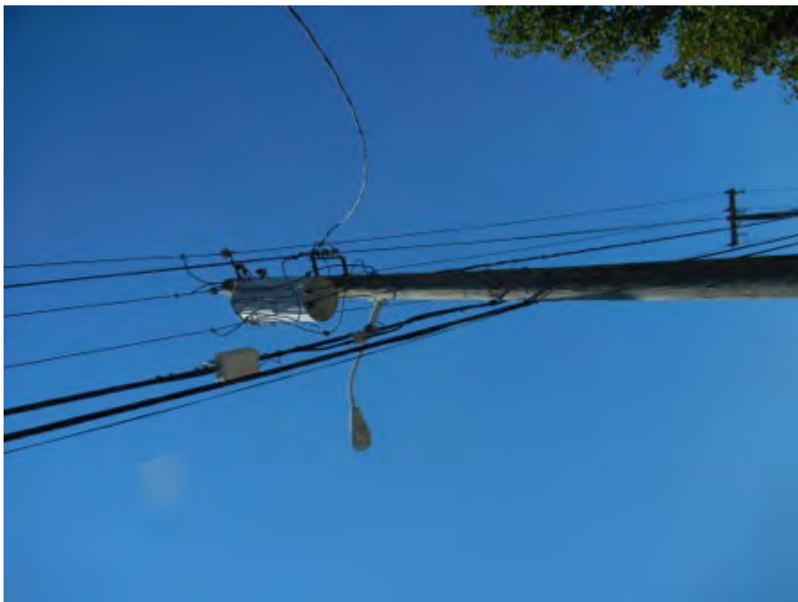
The pole-mounted transformer at the property.
