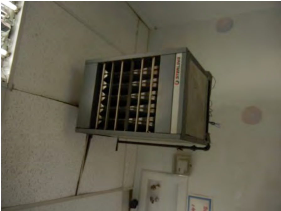
A natural gas ceiling heater at the property.
