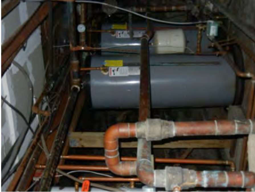
Hot water tanks at the property.
