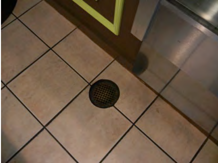
A floor drain at the property.
