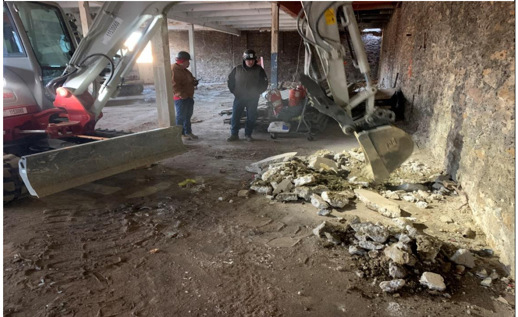
Photo 1 – View of slab removal to excavate a test pit along the northern wall on the first floor
