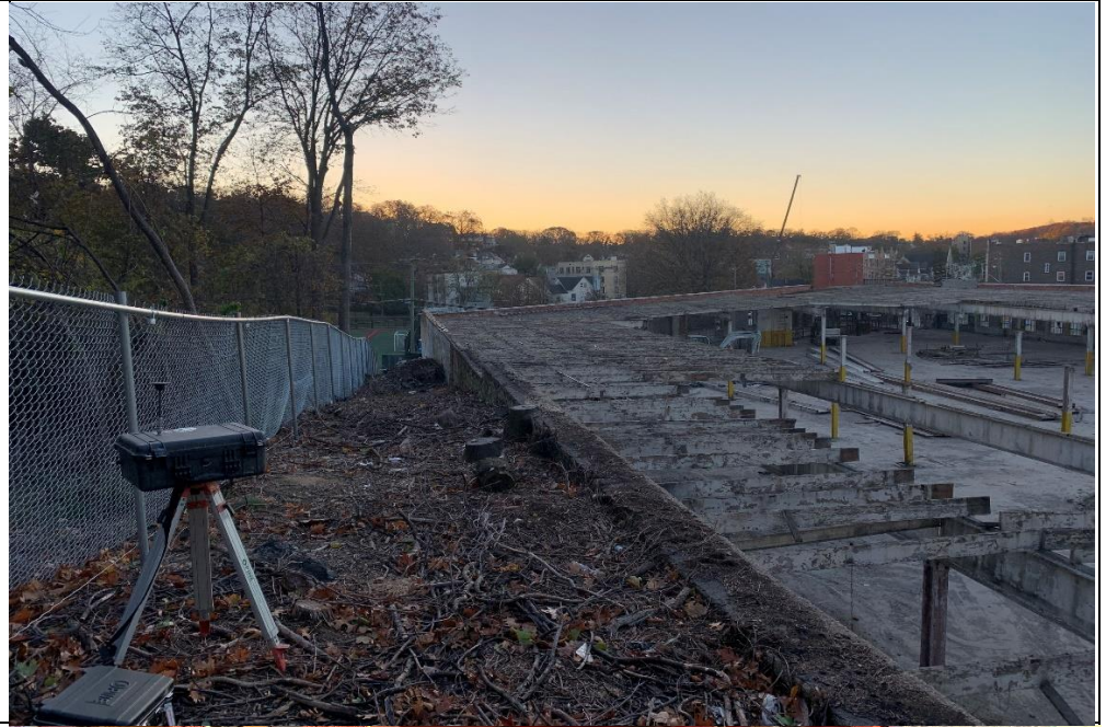
Photo 3 – Down wind CAMP unit station
