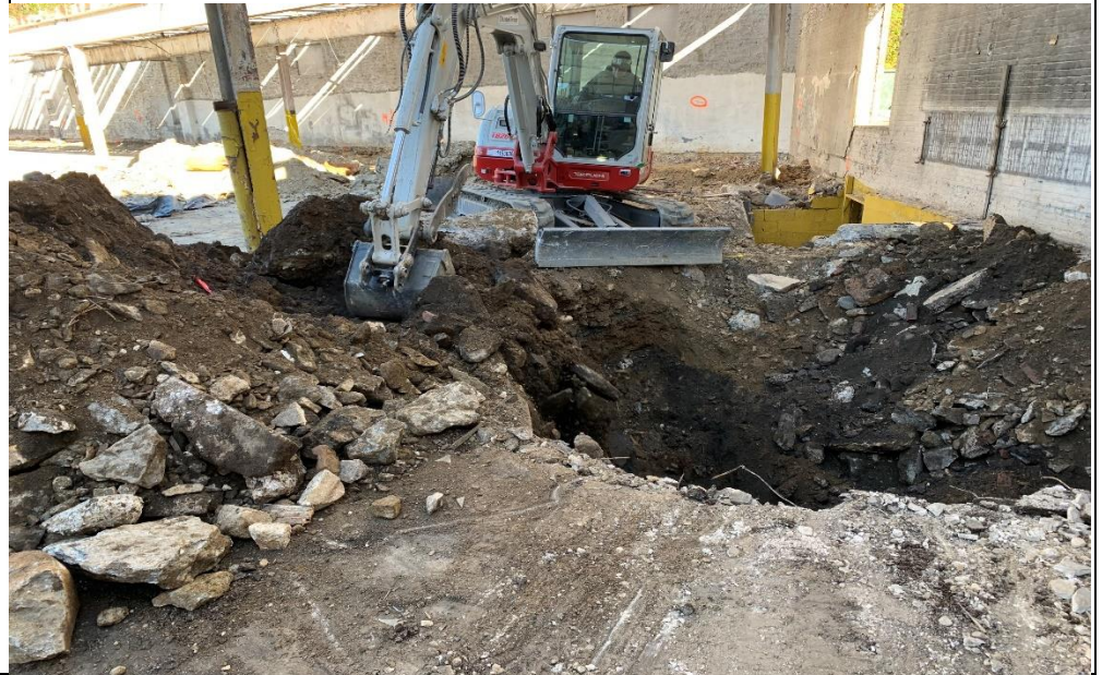
Photo 1 – View of excavation by the staircase and footing on the second floor
