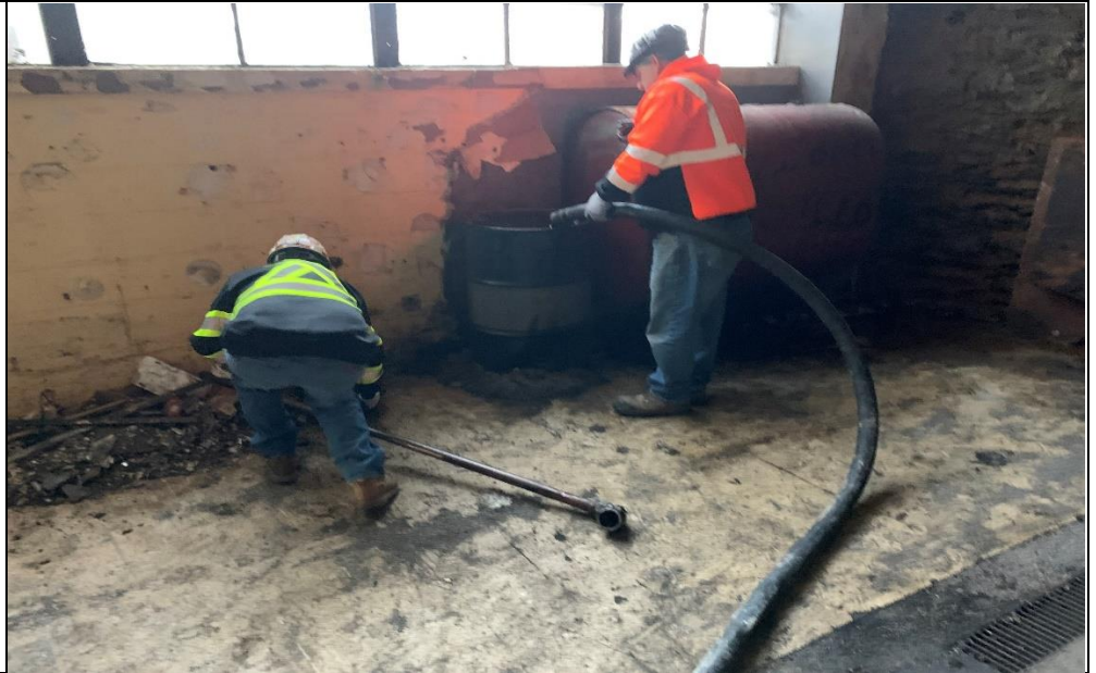
Photo 1 – View of metal drum beside AST being pumped out (waste oil)
