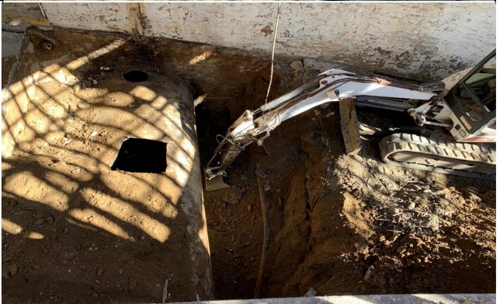
Photo 2 – View of excavation around UST under the ramp, after it was pumped and wiped
