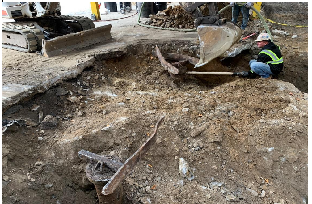
Photo 3 – View of two pistons uncovered post excavation. Fluid pumping on western most piston is visible
