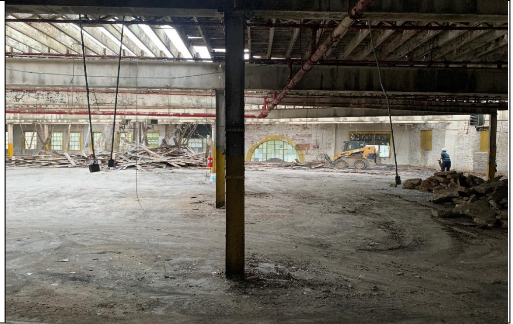
Photo 4 – Wooden panels from roof piled up
