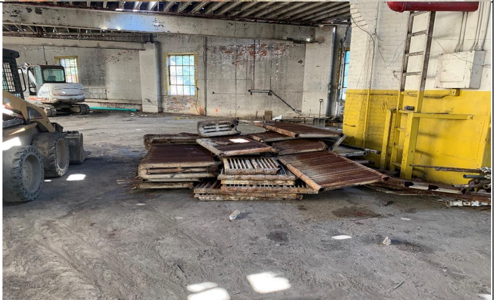
Photo 2 – Pile of radiators (2 nd floor)
