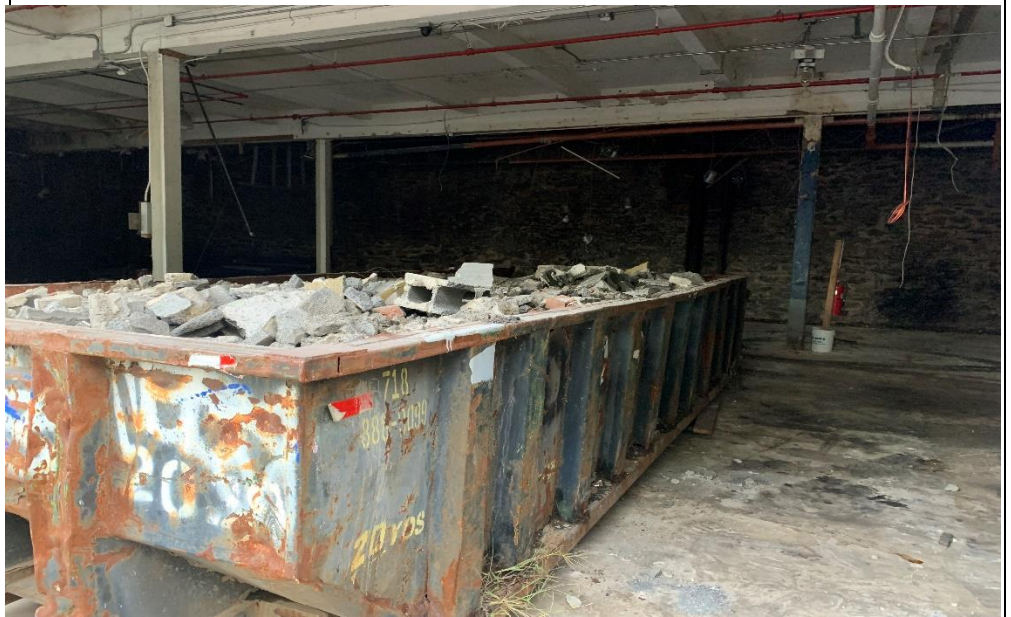
Photo 1 – View of cinder and brick rubble container before loadout (1 st floor)
