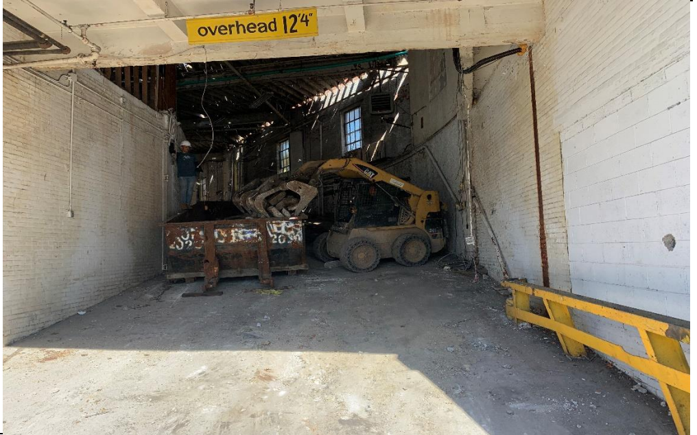
Photo 4 – View of broken slab being loaded into a container on the ramp
