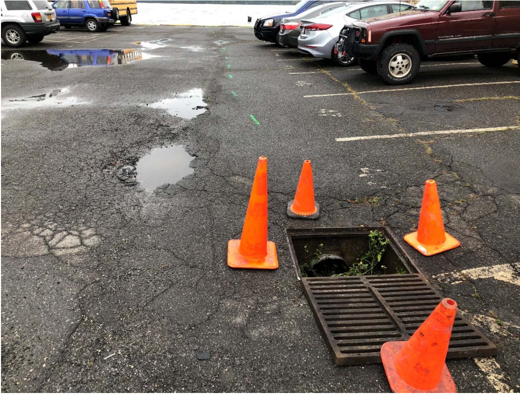
Photograph No. 1: Photograph of storm drain SD-1, which was confirmed to discharge into the Hudson River (facing west).
