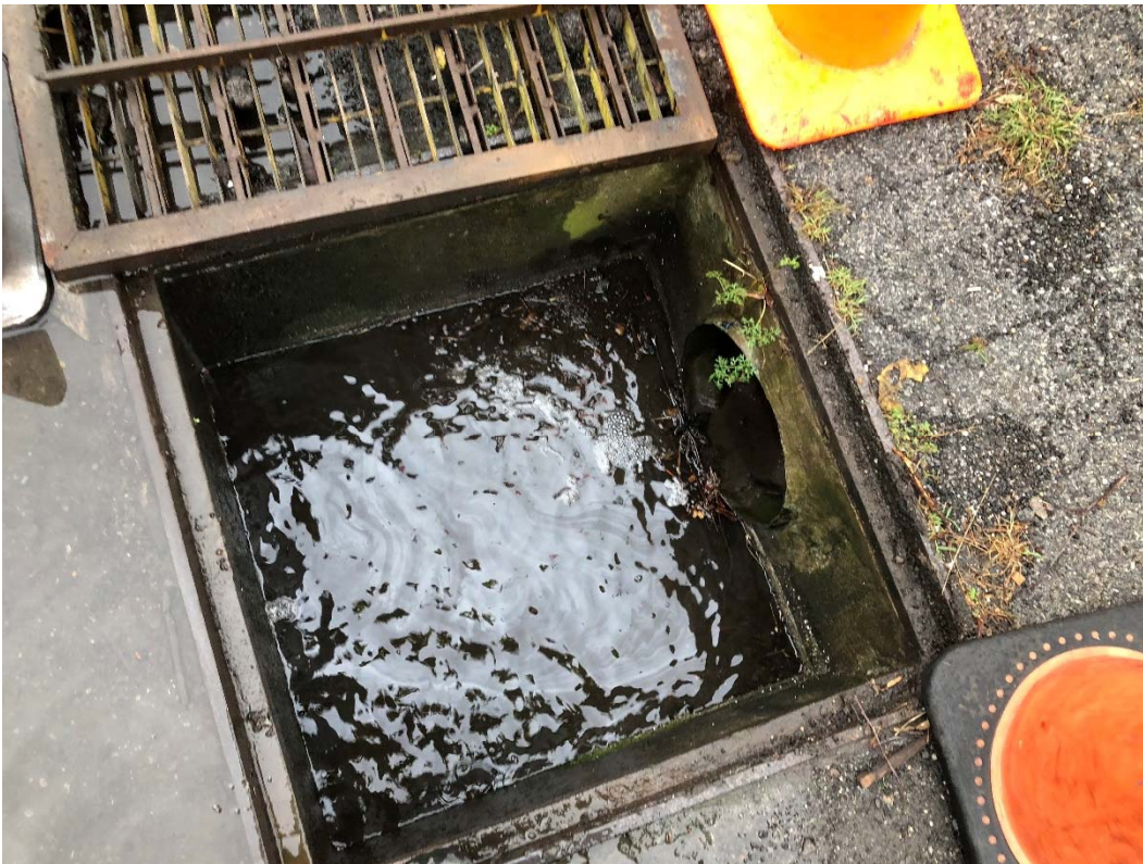
Photograph No. 2: Photograph of storm drain SD-2 located on the southwestern portion of the subject property.
