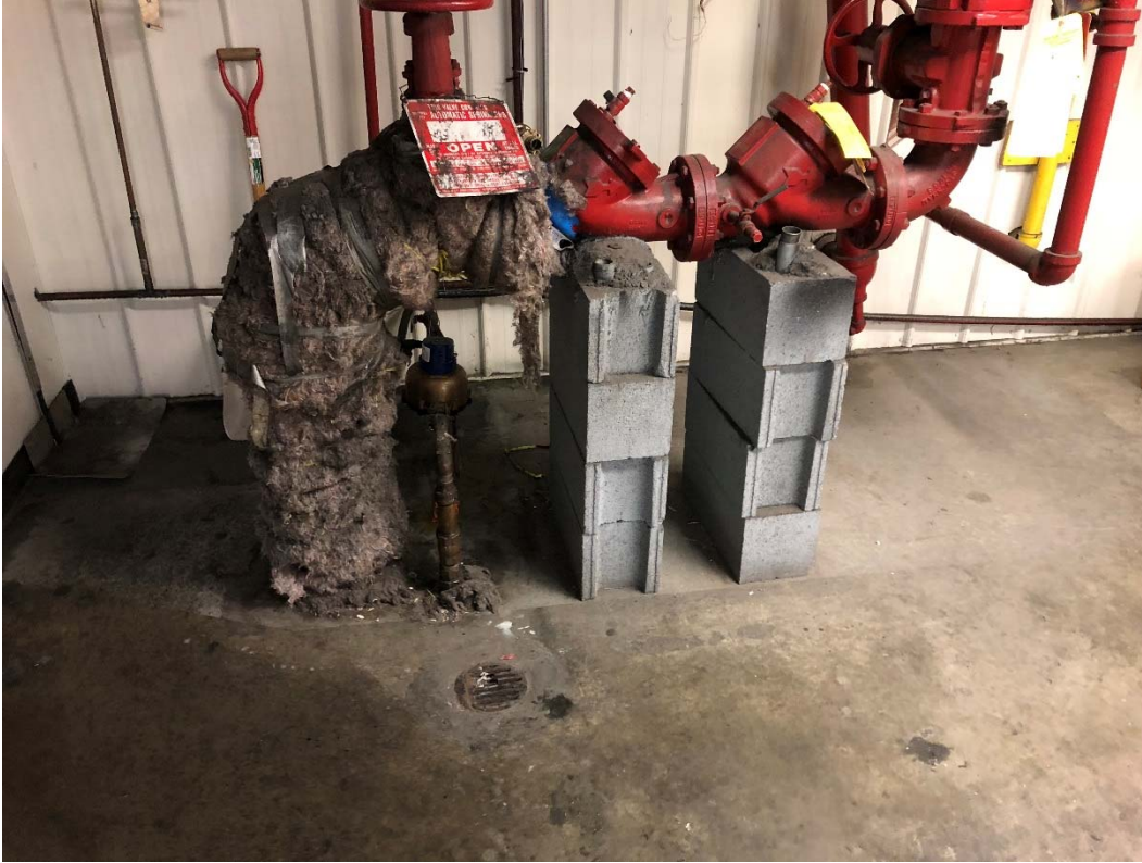
Photograph No. 3: Photograph of the hard-piped interior floor drain located within the eastern portions of Building D.
