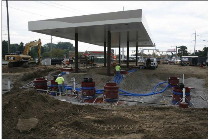
1. Construction of a gasoline service station showing the Underground Storage Tanks and product lines
