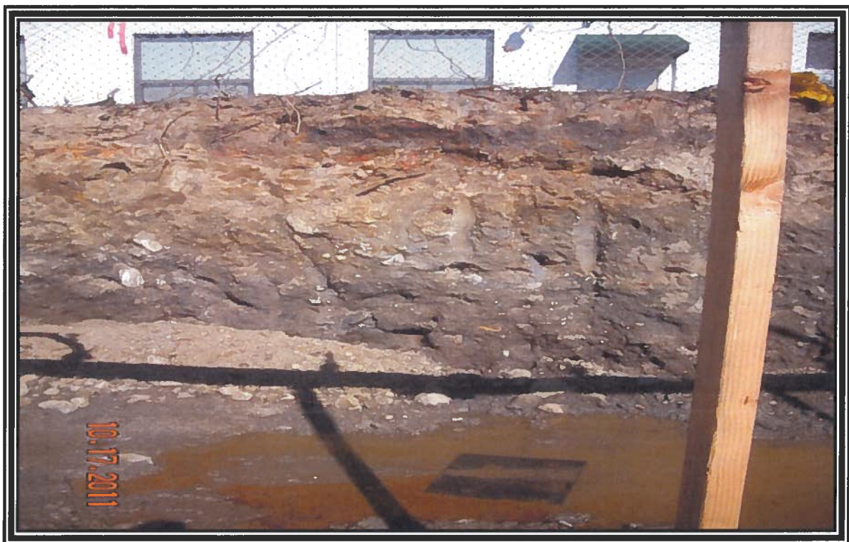
Photograph taken of free-phase product entering the excavation along the eastern sidewall
