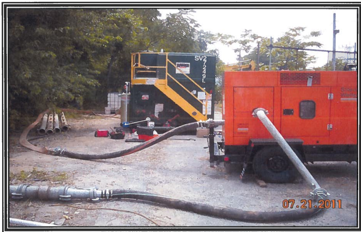
Photograph taken of the on-site dewatering system (pump and frac tank)
