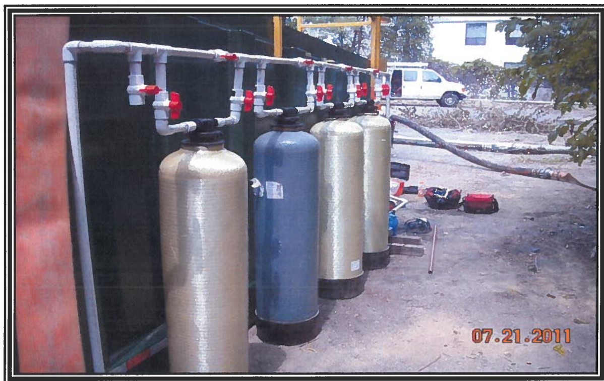
Photograph taken of the carbon filtration installed on the dewatering system discharge vessels
