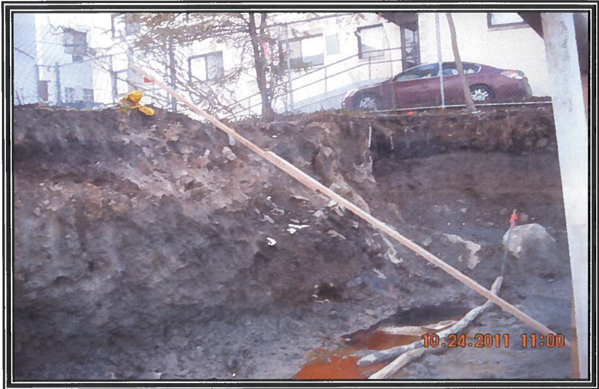
Photograph taken of free-phase product entering the excavation along the eastern sidewall
