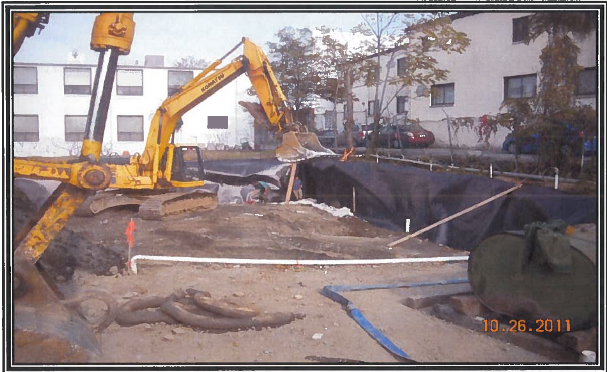
Photograph taken during backfilling and polyethylene barrier installation along the eastern and southern sidewalls
