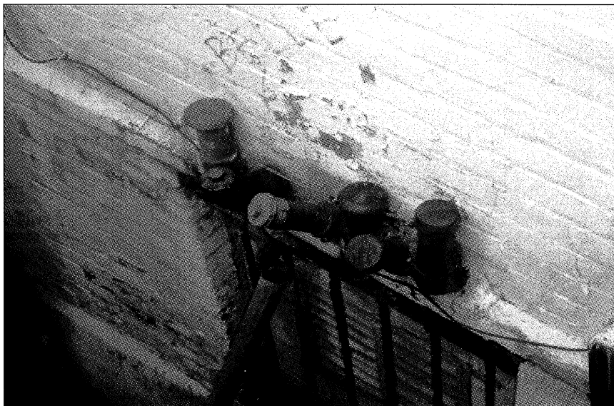
FUEL OIL FILL PORTS AND VENT PIPES LOCATED AT THE EASTERN EXTERIOR WALL OF BELLE LAUNDRY AND CLEANERS.
