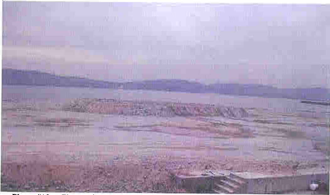
Photo #13 - Clean soil cover -central area. Soil surcharge berm shown in center.
