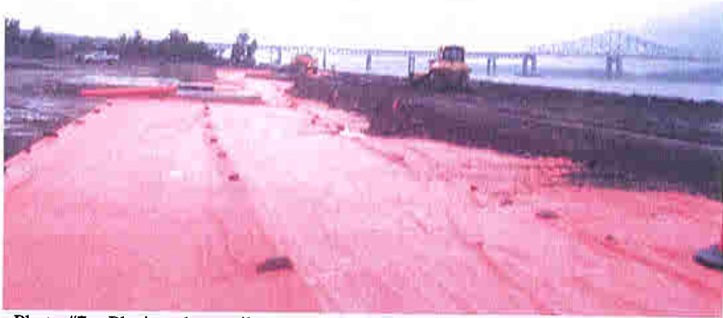
Photo #7 - Placing clean soil cover - central area. Note traffic cone "grade stakes".
