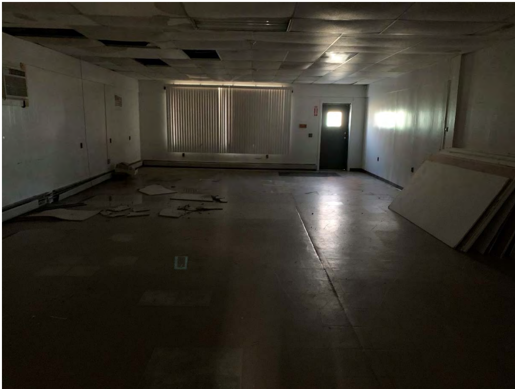
(ACM Joint Compound on Non-ACM Sheetrock Walls in Room 2)
