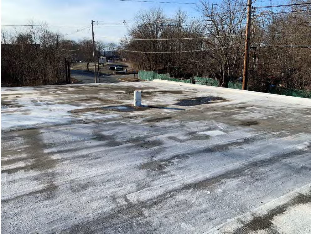
(Roof with Second Layer ACM Built-up Roofing and Second Layer ACM Perimeter Flashing Tar)
