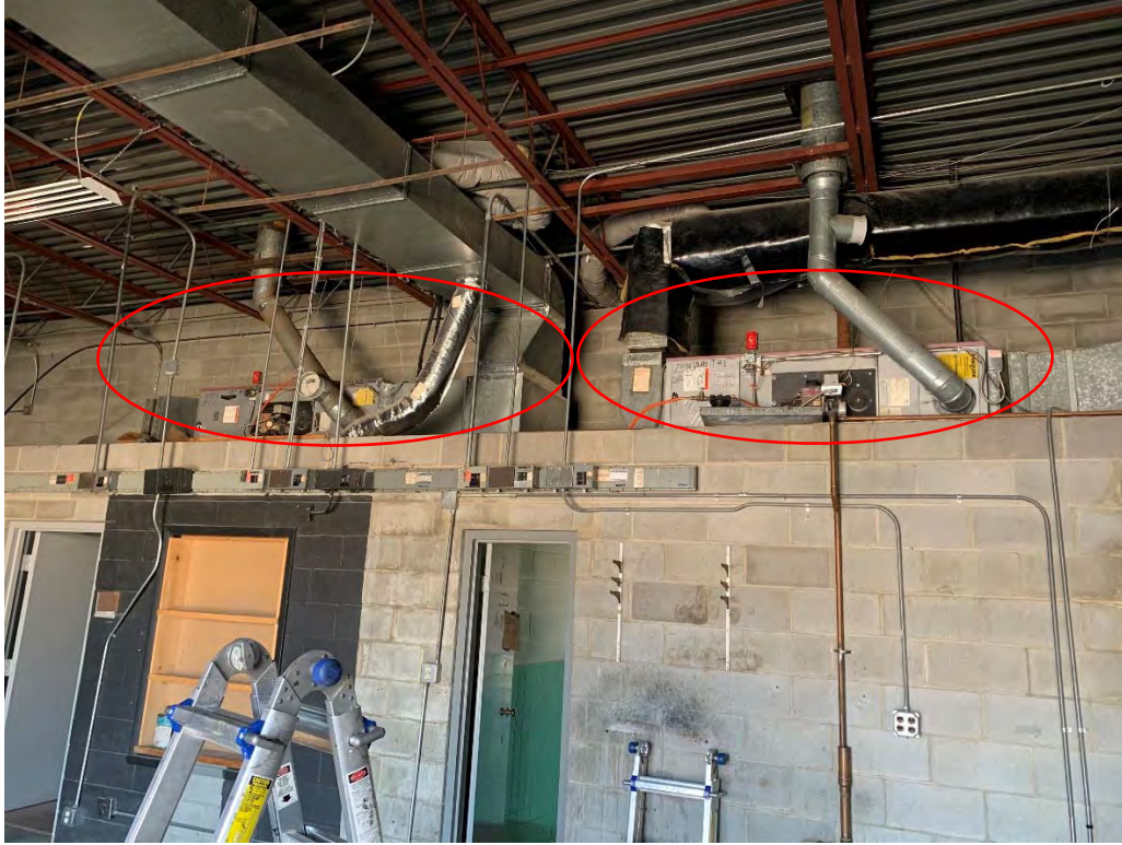
(Circled in Red: Location of Fiber Panel under HVAC Equipment in Garage 2)
