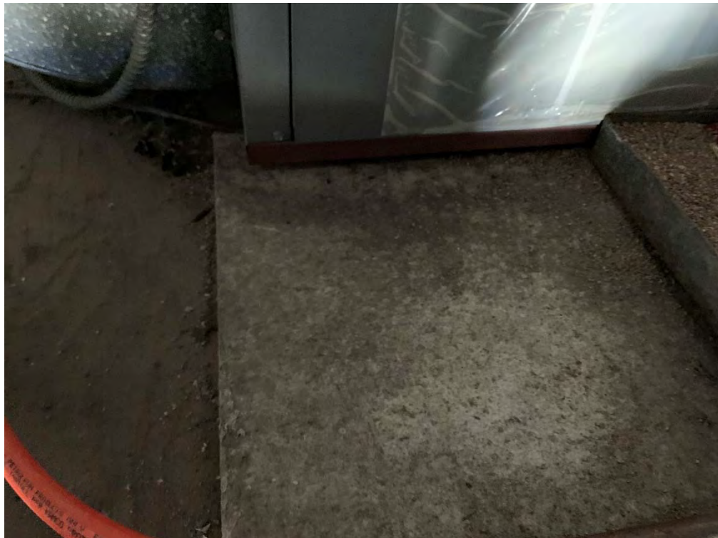
(ACM Fiber Panel Under HVAC Equipment in Garage 2)
