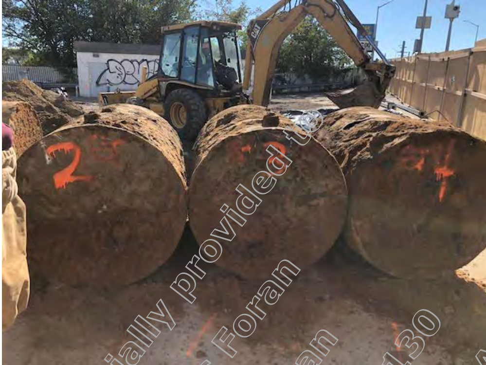
Condition of the remaining three unknown tanks
