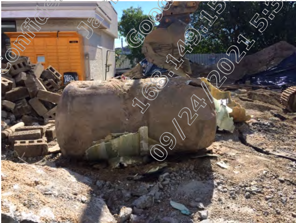
Tank #6 (fiberglass broken away showing concrete)
