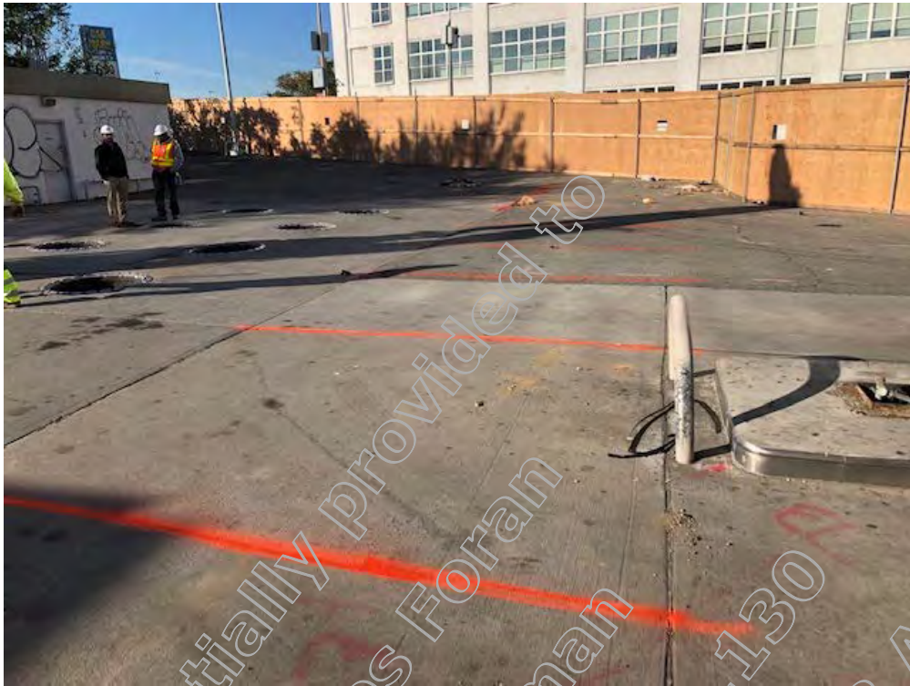
Underground storage tank field area
